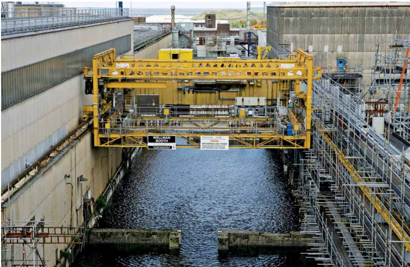
Elevated view of the pond and gantry system
