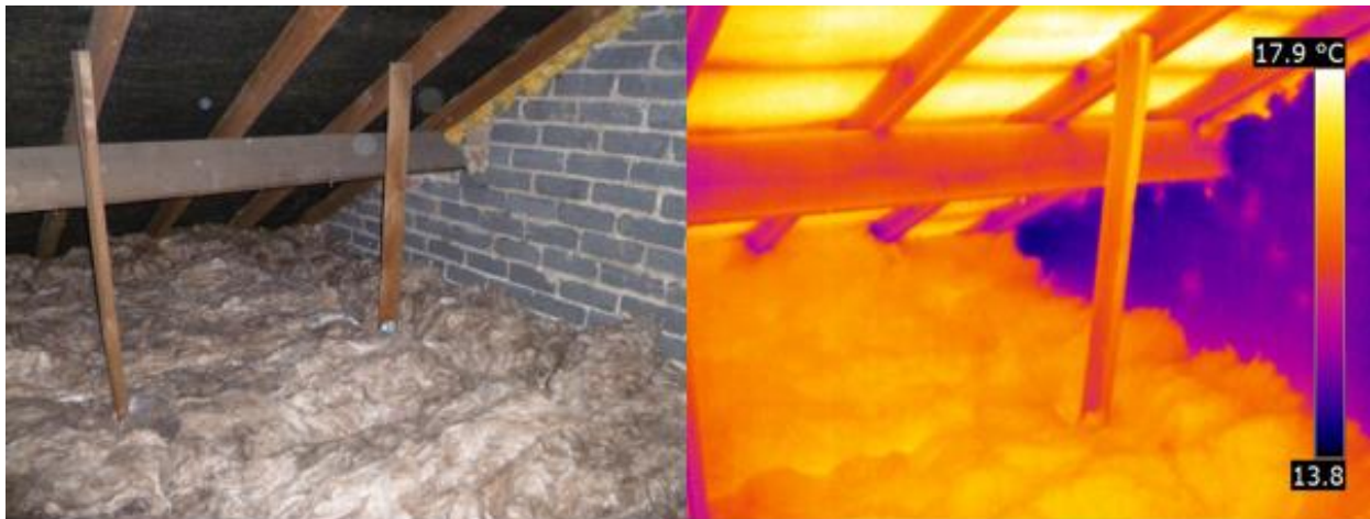
Figure A3: Image and thermogram of the loft space with the retrofit loft insulation fitted
