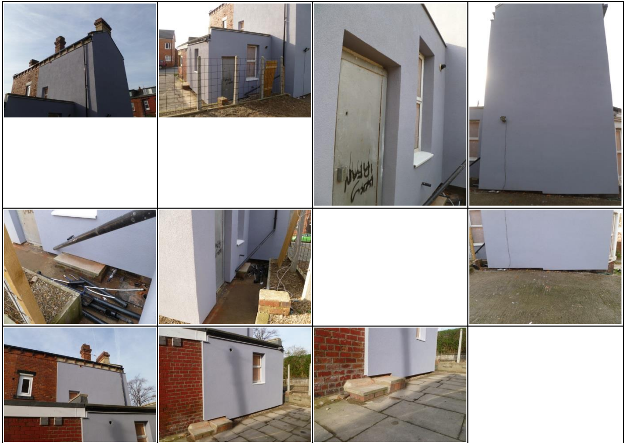
Gaps between wall and EW1?
