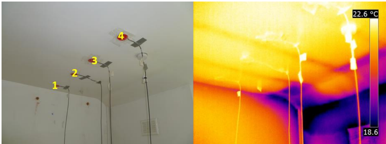
Figure A5: Image and thermogram of the ceiling in bedroom 3 post-retrofit. Numbers 1-4 are the roof HFP identifiers.
