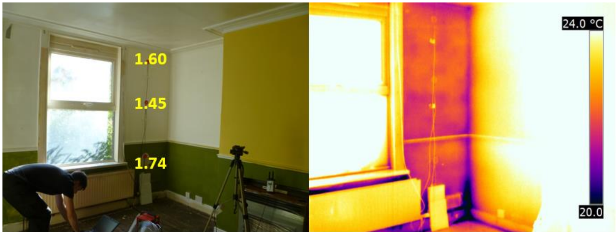
Figure 3: Annotated image and thermogram showing the ground floor pre-retrofit external wall U-value measurements
