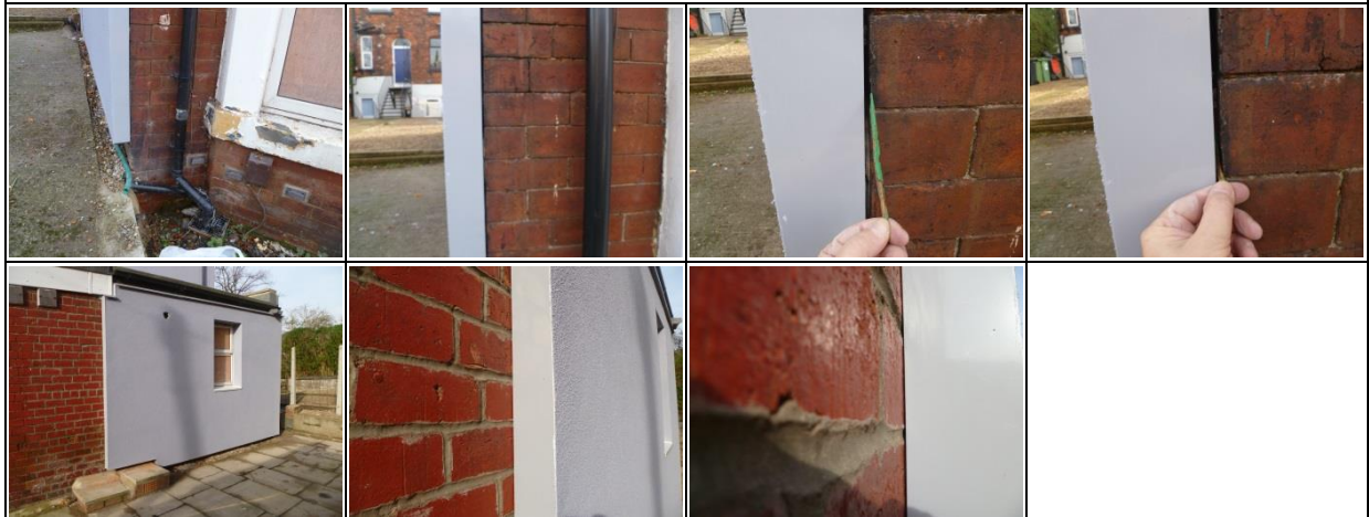
EPS wall beads leaking out of wall vents at rear of building?
