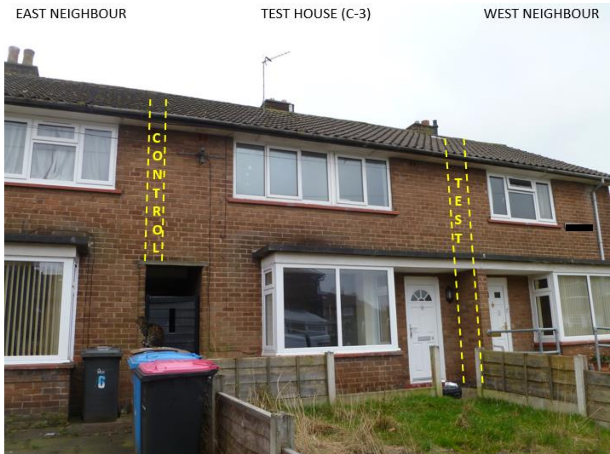
Figure 2: Image of the front of the test house illustrating the location and designation of the party walls
