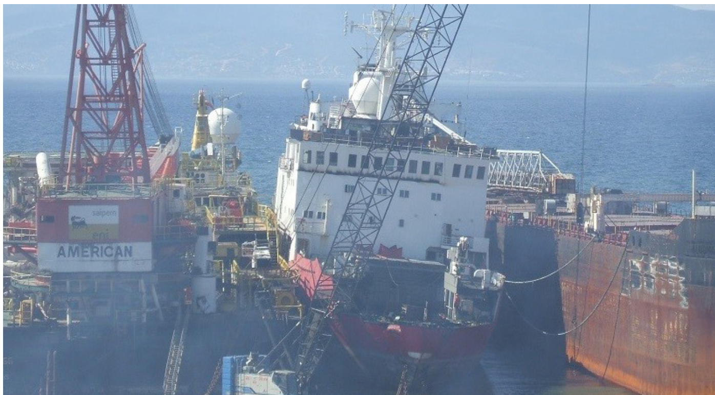
1 July 2016 - First stages of dismantling of the keel section. Heavy Machinery is used to remove large pieces of the vessel for processing.
