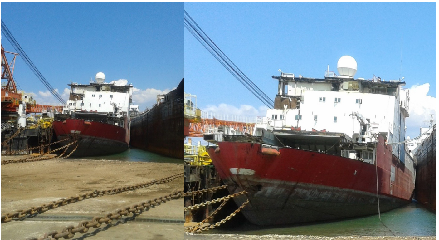
7 July 2016 - The vessel is dismantled from 'top to bottom' while afloat and from 'bow to stern' on the dry slipway.
