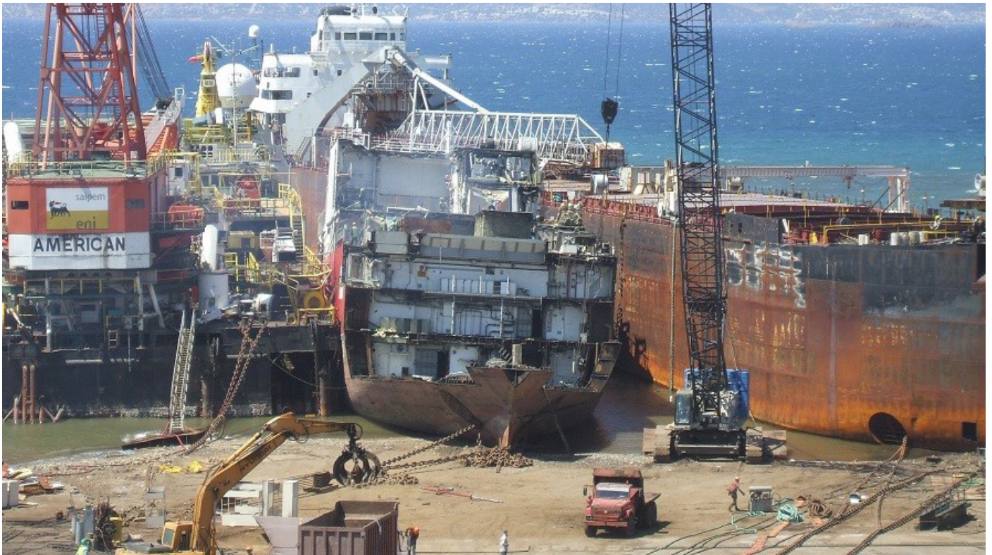
19 July 2016 - Showing remains of the engine room. Heavy lift cranes are used to remove large parts of the machinery. Secondary cutting and further processing and material separation takes place.
