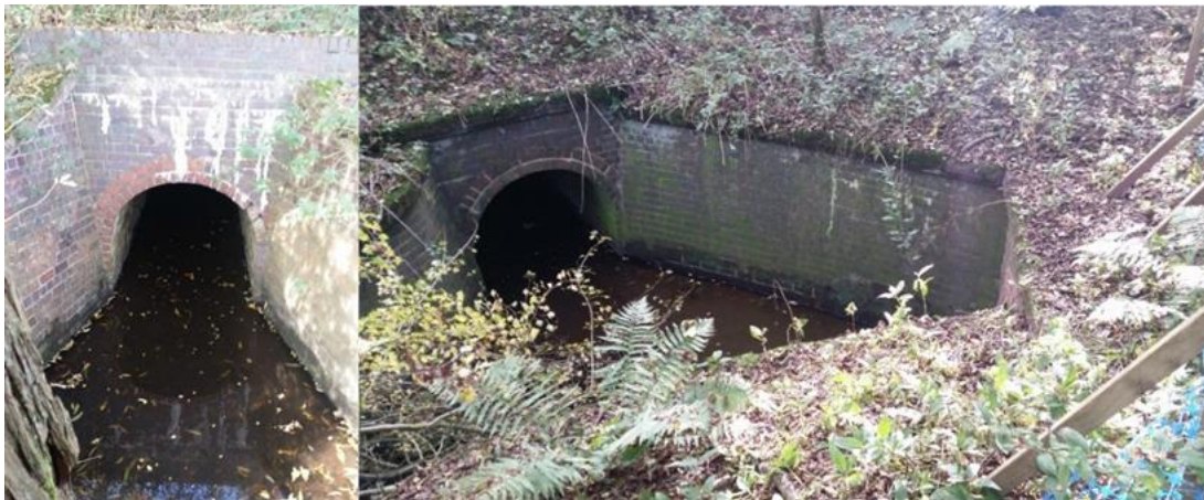
Figure 3: LeaCulo1 outlet and Culvo6 inlet
