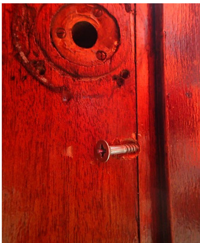
Figure 15: The method of securing a toilet cubicle door using screws through the door and frame
