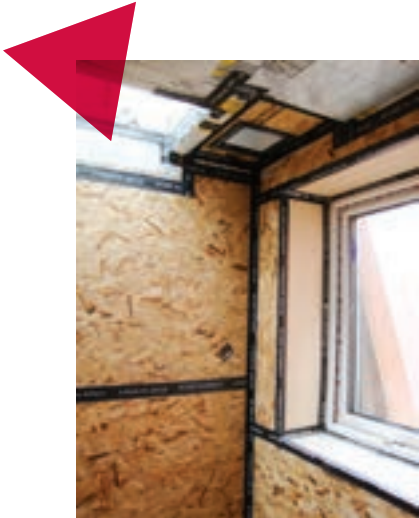
Attention to detail can result in excellent airtightness [North Belfast, case study 1, House 1, page 44].
