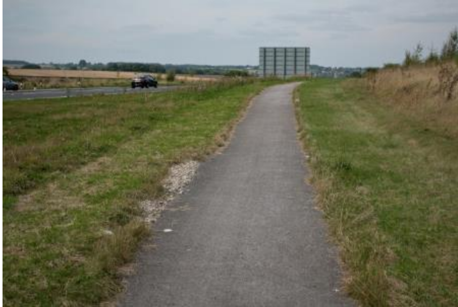
Figure H.5 Wattle Syke to Wetherby Grange NMU route: cut off drainage has been provided and the ponding issue appears to have been resolved
