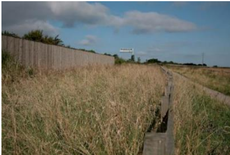
Figure 5.9 The environmental barrier replacing the noise bund adjacent to the southbound carriageway, directly north of Farfield House remains unplanted (top and bottom)
