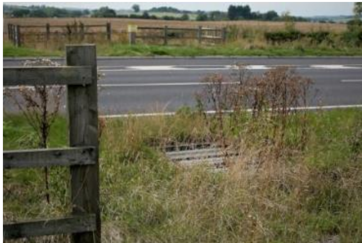
Figure 5.21 Vegetation and construction debris within the equestrian corral on the LAR just north of Wattle Syke Roundabout
