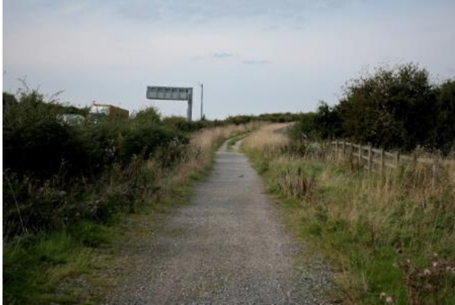
Figure H.9 York Road North, east side re-profiled NMU route: no evidence of ponding was observed
