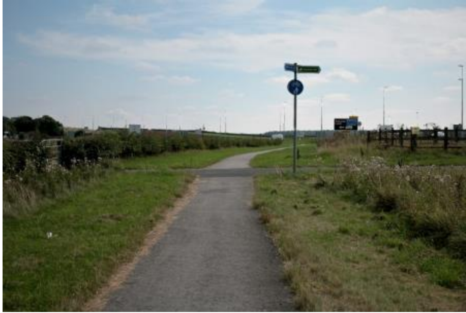
Figure H.4 Wattle Syke north: the ponding issues adjacent to the farm access appear to have been resolved
