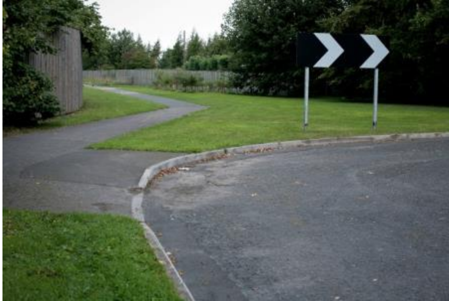
Figure H.3 Fairfield House Junction: the ponding issue appears to have been resolved with surface runoff directed into the drain.
