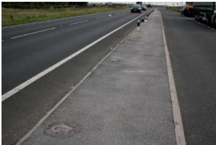
Figure 5.24 Demarcation posts at the lay-by on the LAR between Wattle Syke and Wetherby: missing posts on the splitter island (top) and damaged posts in the verge (bottom)
