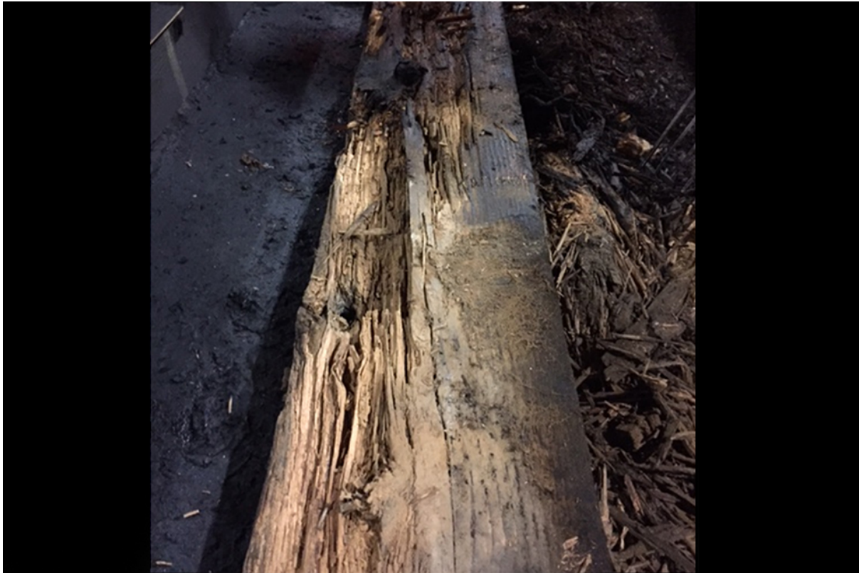
Underside of decayed right-hand timber (image courtesy of Network Rail)
