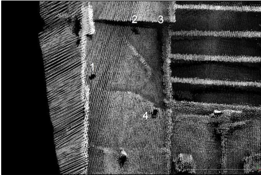
Fig. 13 Holes in Deck Plate shown in the 2015 point cloud
