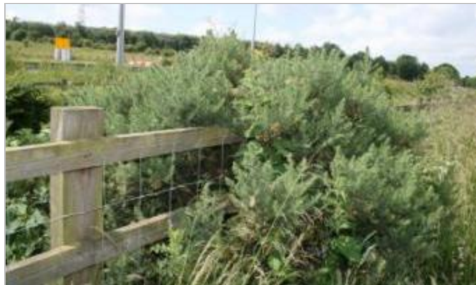
Figure 5.17 Example of weeds found within balancing ponds and culverts
