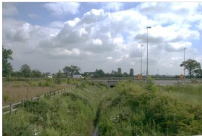
Figure 5.18 Overgrown vegetation in Rockcliffe Beck culvert
