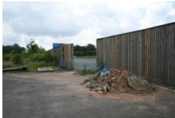
Figure 5.4 Missing acoustic barriers at Todhills
