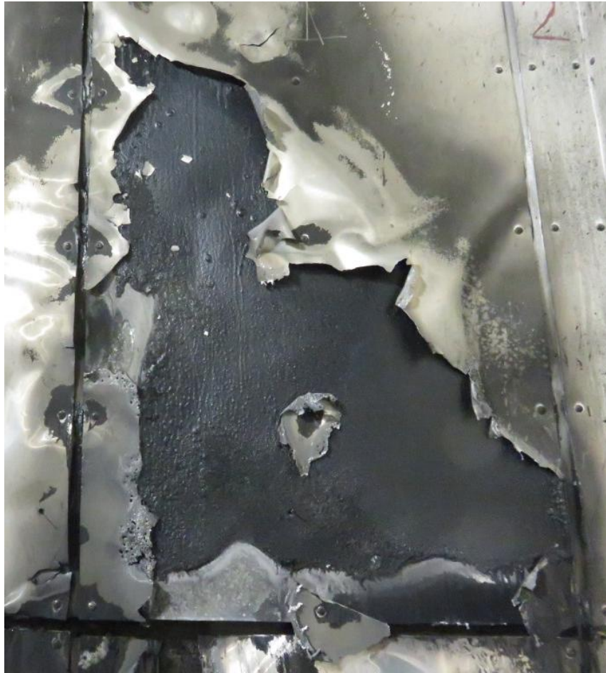
Figure 25. Close up of panel 2C (approximately 4600mm above the top of the combustion chamber) showing melted aluminium outer face with intact PE core material.
