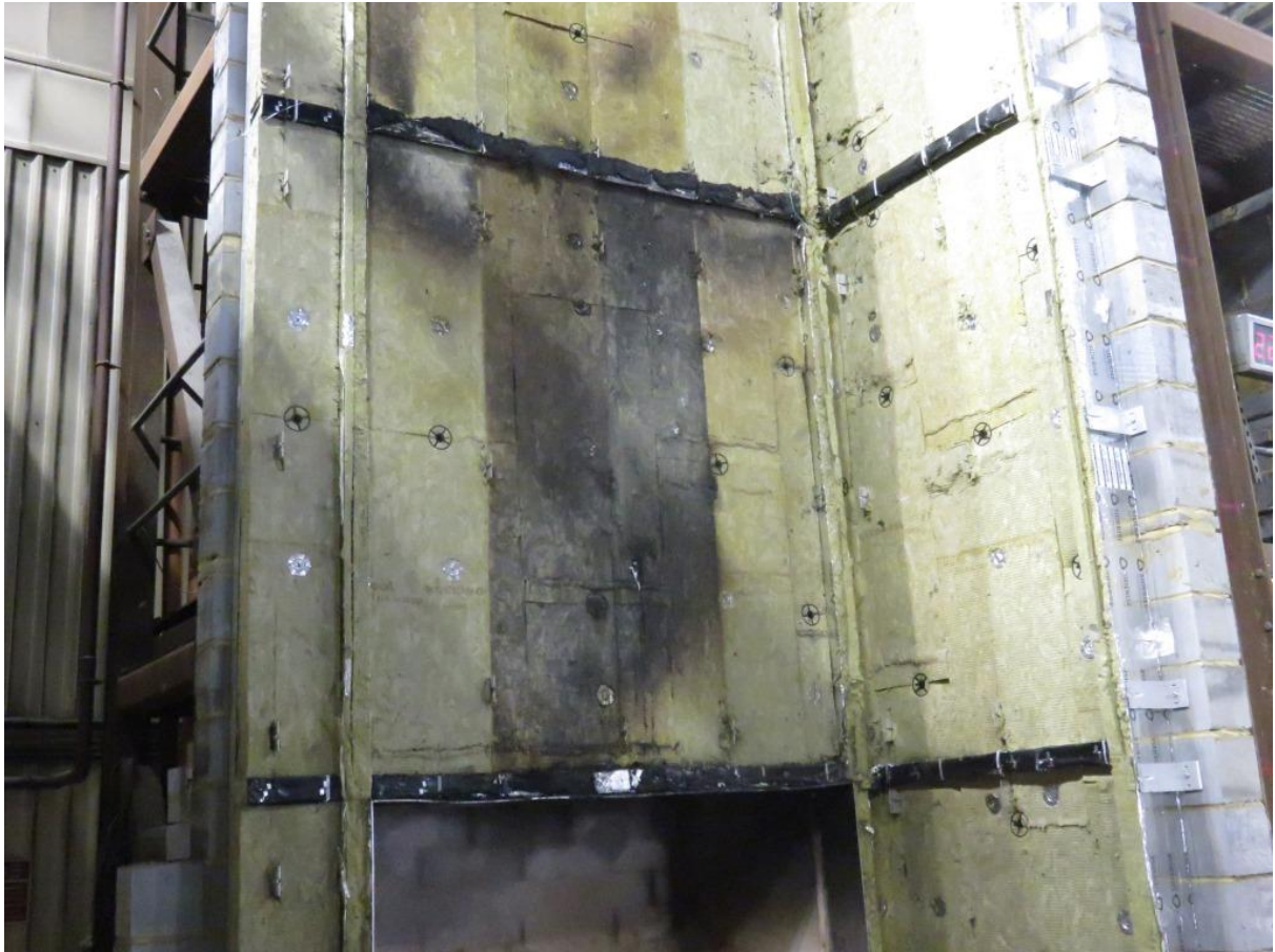
Figure 29. Cladding system beneath ACM panels and rail substructure between the first and second horizontal cavity barrier (approximately 0-2400mm above combustion chamber).
