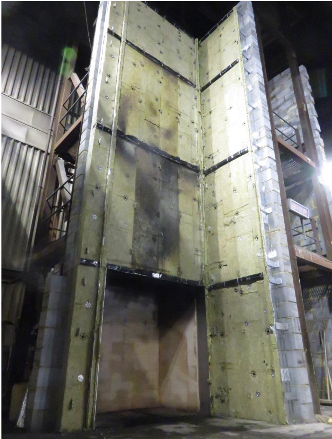
Figure 28. Full height photograph of cladding system following removal of ACM panels and rail substructure.
