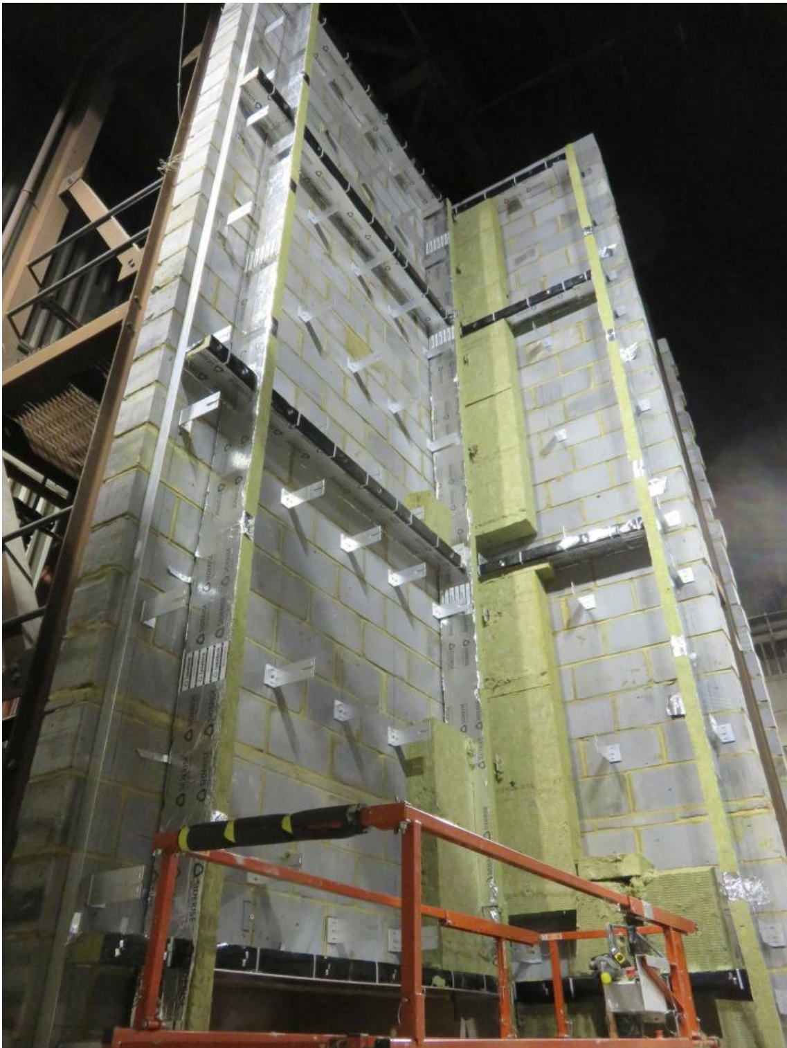
Figure 5. Horizontal intumescent cavity barriers fixed through the entire depth on face turned steel brackets, fitted between vertical cavity barriers.
