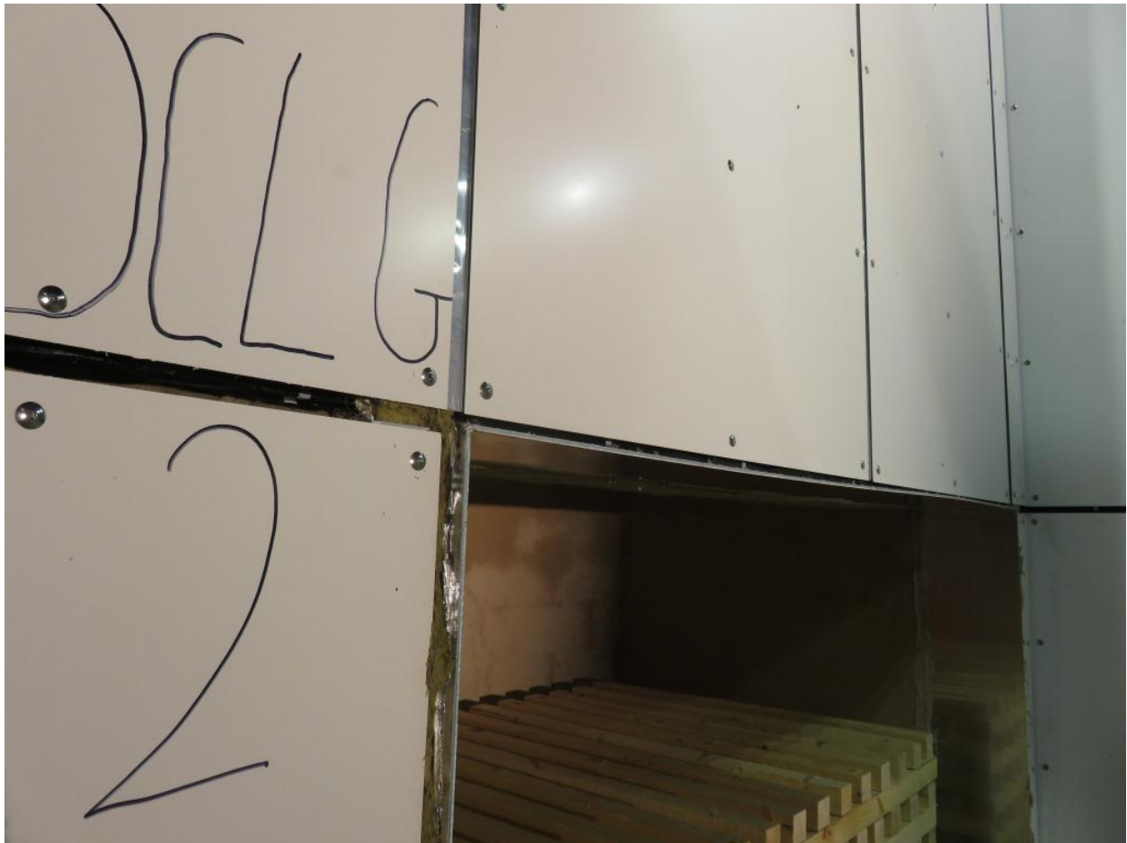
Figure 10. Detail at corner of combustion chamber opening. Panels riveted in place and nominal 20mm vertical gap left for ventilation purposes.
