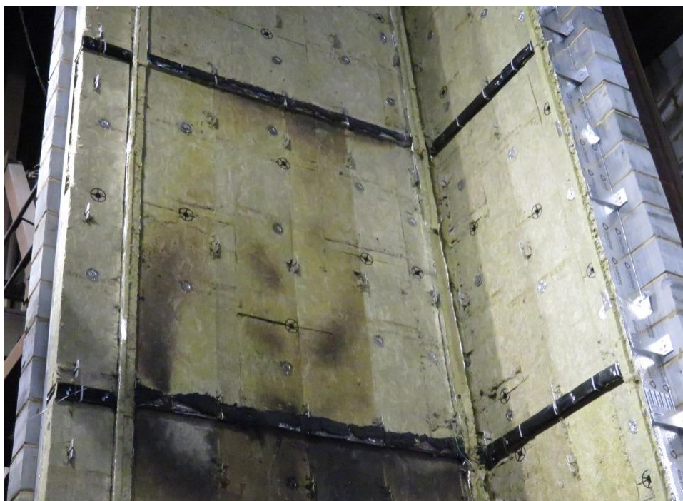
Figure 30. Cladding system beneath ACM panels between the second and third horizontal cavity barrier (approximately 2400-4700mm above combustion chamber).
