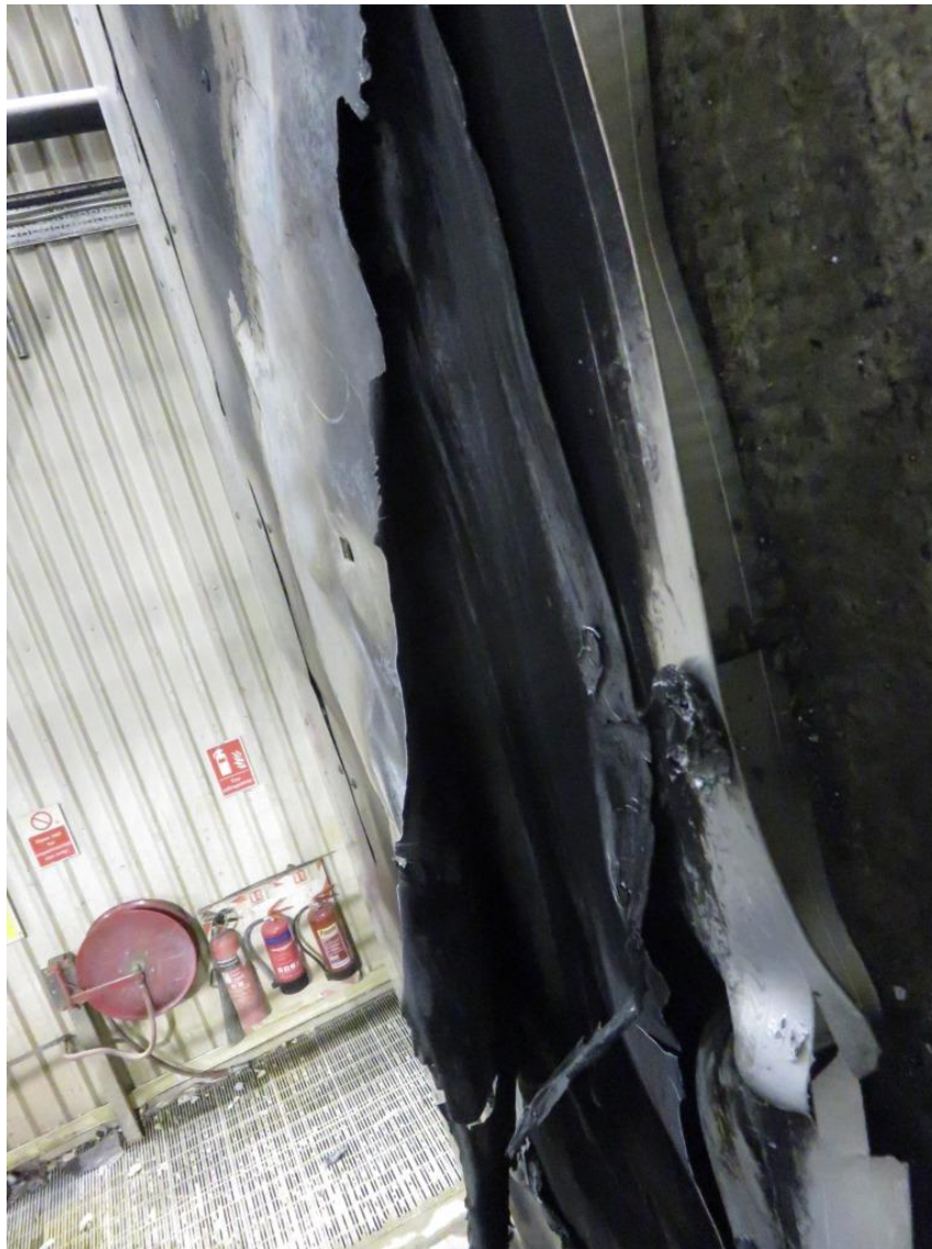
Figure 24. View between distorted aluminium layers of panel 1D (approximately 1000mm above the top of the combustion chamber) showing absence PE core material.
