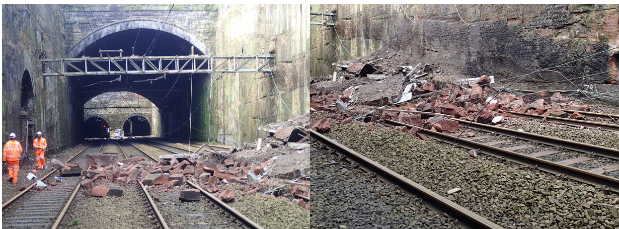
Figure 3: The debris on the track following the wall collapse
