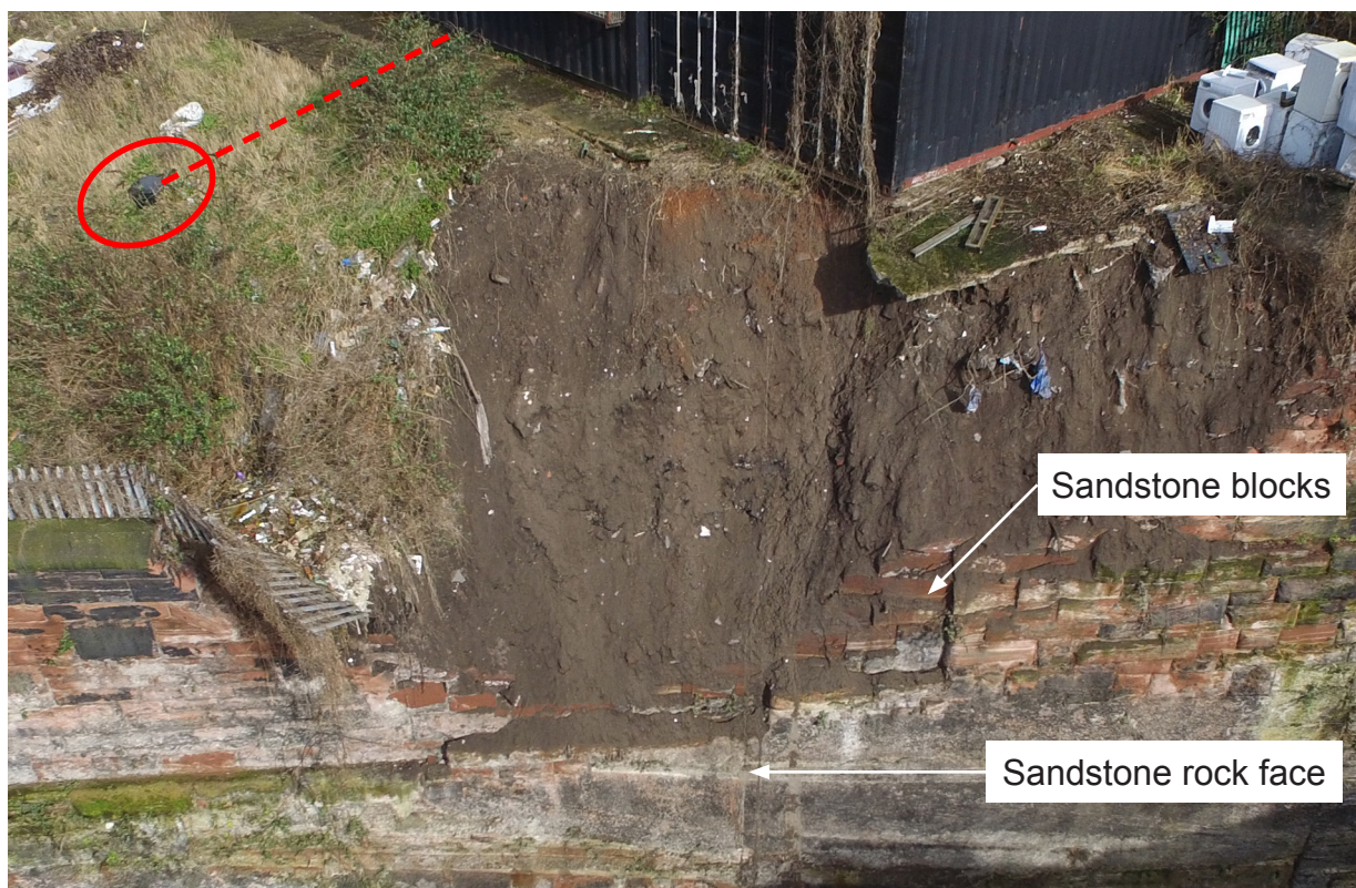
Figure 12: The upper part of the cutting wall following the collapse (red circle indicates a drain chamber - see paragraph 39)
