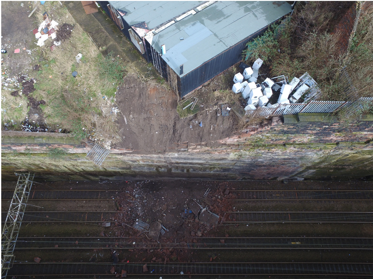
Figure 2: The cutting following the collapse of the retaining wall
