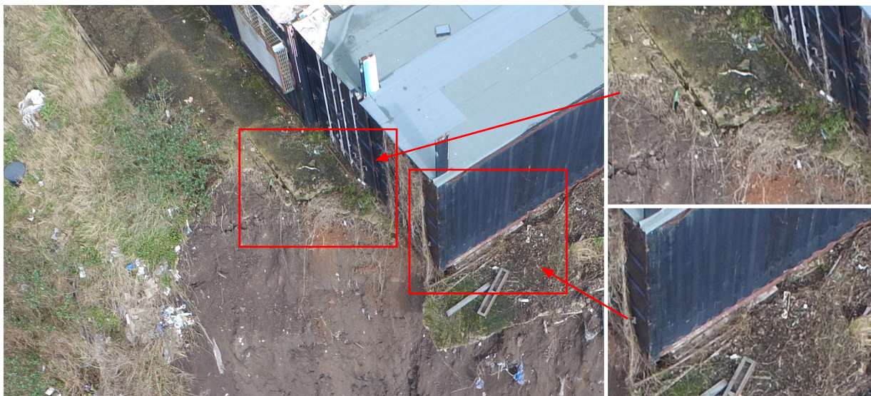
Figure 14: The soil embankment following the collapse showing pre-existing cracks in the concrete slab
