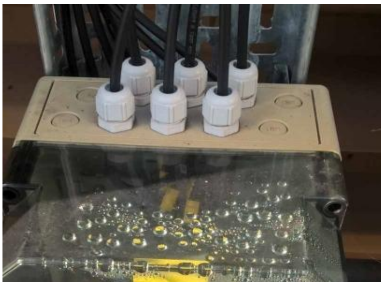
Figure 8: Water can be seen inside this enclosure, even though only one cable passes through each gland.
