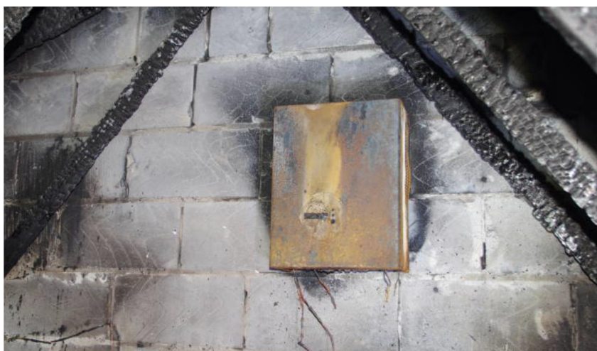
Figure 13: Inverter fire with clear burn patterns showing this as the source of the fire.
