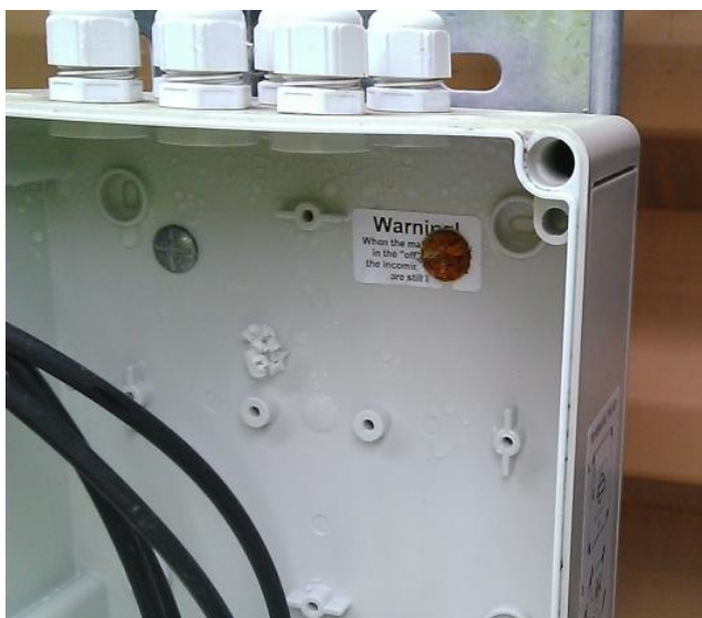
Figure 9: Rear of isolator enclosure drilled through for mounting screws. Note that the screw on the right hand side is rusty, indicating water ingress.
