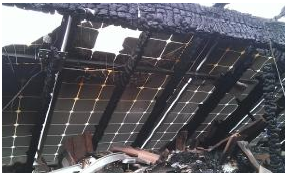
Figure 3: Example burnt-out roof with parts of the PV system intact.
