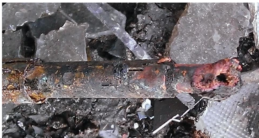
Figure 12: Example of DC connector contact that has been subject to electrical arcing. The right hand end has been melted.
