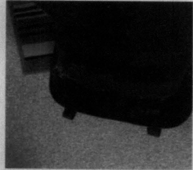
Typical mould growth on items stored within cupboards
