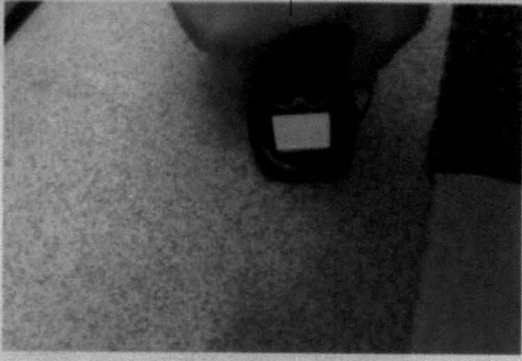
Wet vinyl flooring in kitchen
