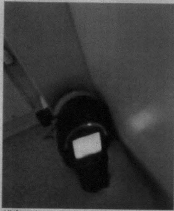
High moisture reading in Kitchen
