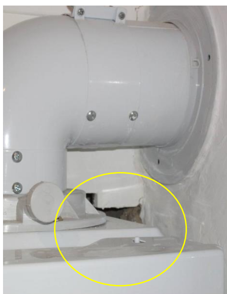
Figure 7: Large gap left at back of new boiler allowed significant amount of air leakage
