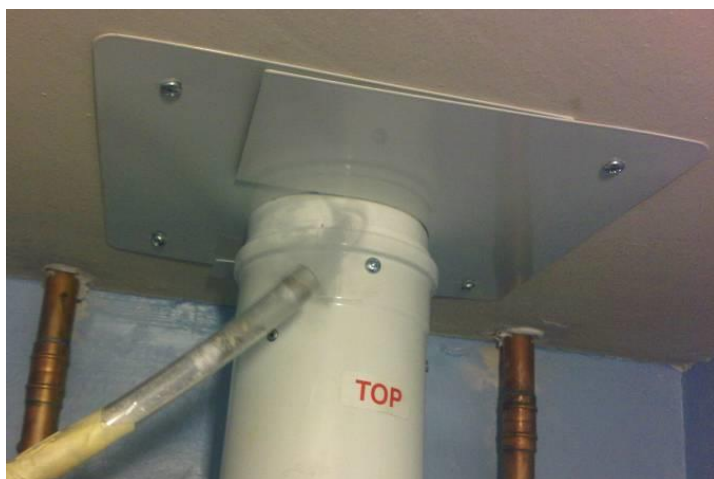
Figure 3: Additional leakage routes found post-refurbishment around central heating pipes
