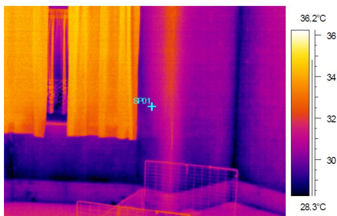
Figure 8: Cold walls in front room pre-refurbishment
