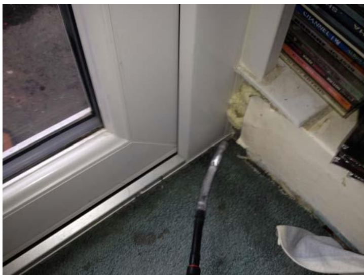
Figure 4: Example of poor window sealing using expanding foam following a window replacement
