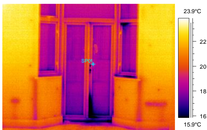
Figure 16: Thermal image of patio doors
