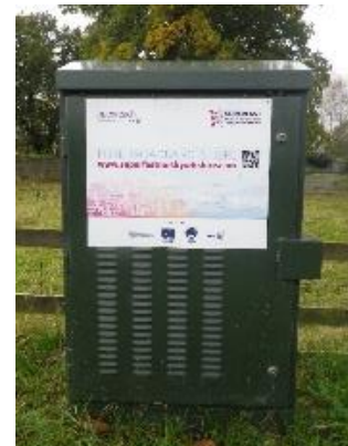
A second generation (superfast) cabinet
