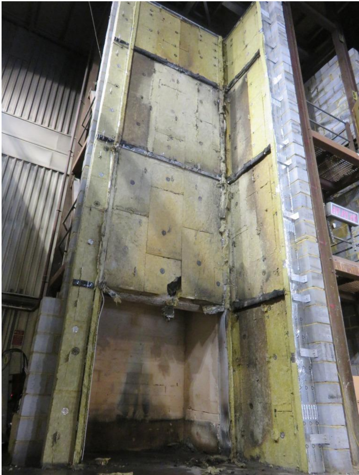
Figure 31. Full height photograph of cladding system following removal of ACM panels and rail substructure.
