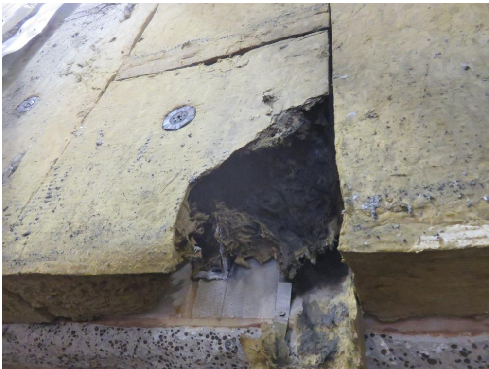
Figure 28. Close up of detached section of stone wool insulation directly above the combustion chamber.
