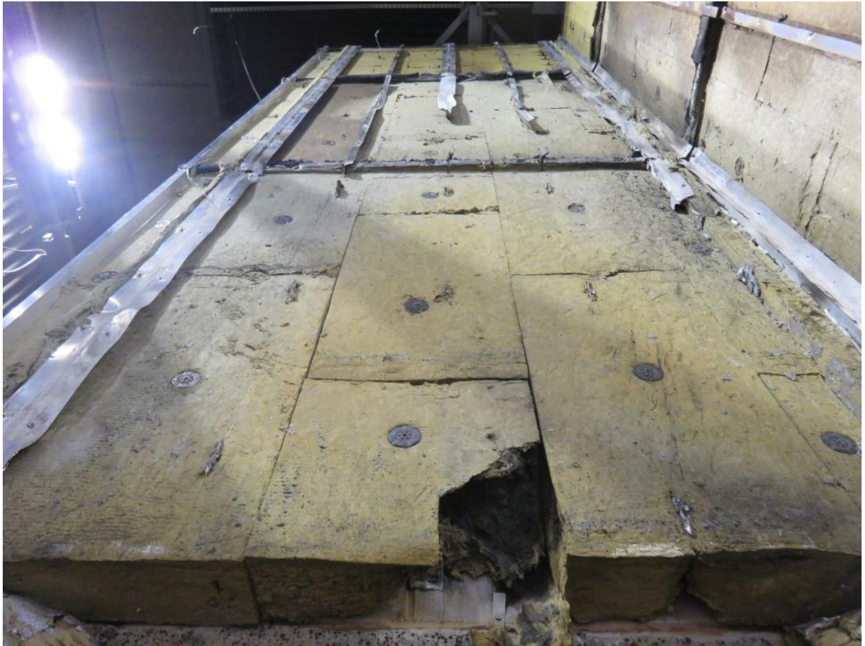
Figure 30. Damage to cladding system beneath ACM panels directly above the combustion chamber.
