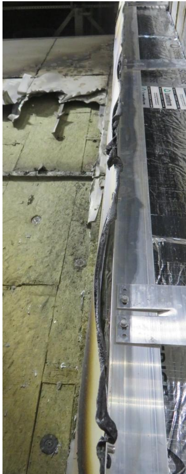
Figure 26. Close up of ACM panel edges showing melted core filler material.
