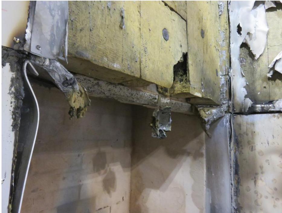
Figure 27. Close up of melted window pod and collapsed horizontal cavity barrier directly above the combustion chamber.
