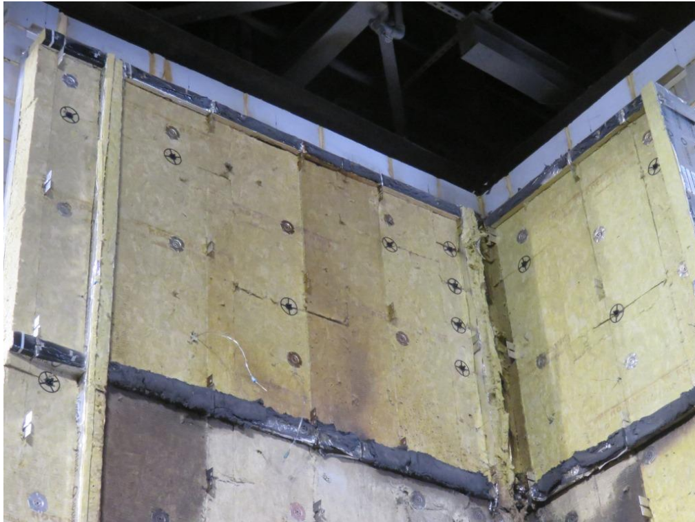
Figure 35. Cladding system beneath ACM panels between the third and fourth horizontal cavity barrier (approximately 4700-6400mm above the combustion chamber).
