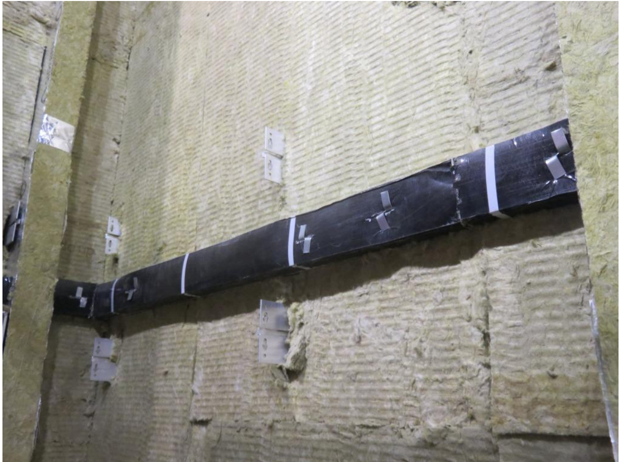
Figure 4. Horizontal intumescent cavity barrier fixed through the entire depth on face turned steel brackets, fitted between vertical cavity barriers.
