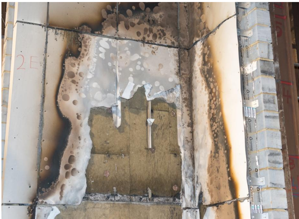
Figure 24. Second row ACM panels (approximately 2300mm-4600mm above combustion chamber).
