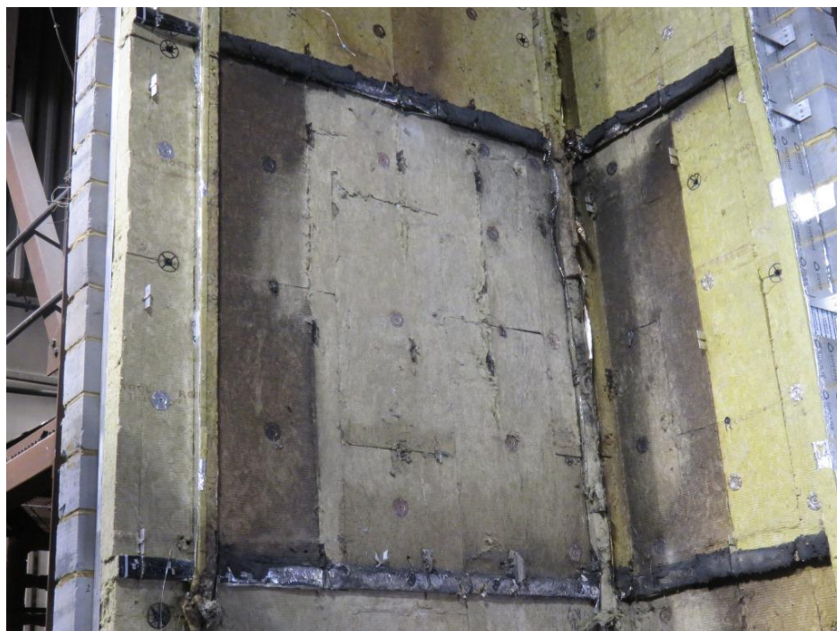
Figure 34. Cladding system beneath ACM panels between the second and third horizontal cavity barrier (approximately 2400-4700mm above combustion chamber).
