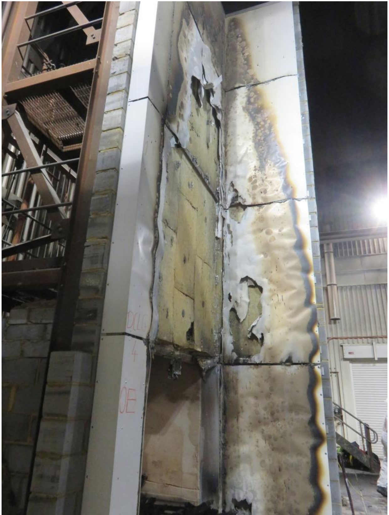
Figure 22. Full height photograph of wing wall post-test.
