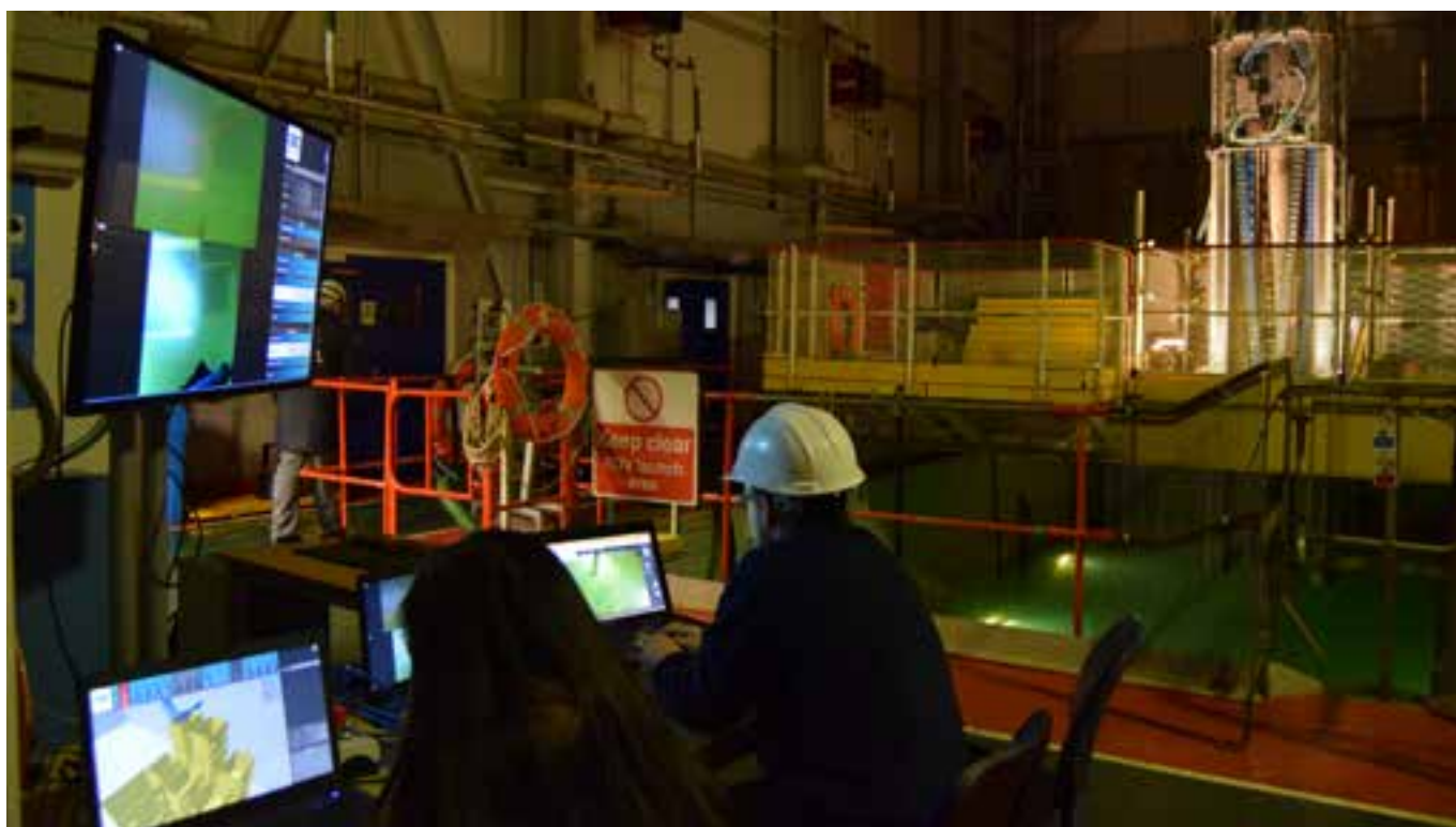
Control desk with OCR operators carrying out commissioning tests with the snakearm
