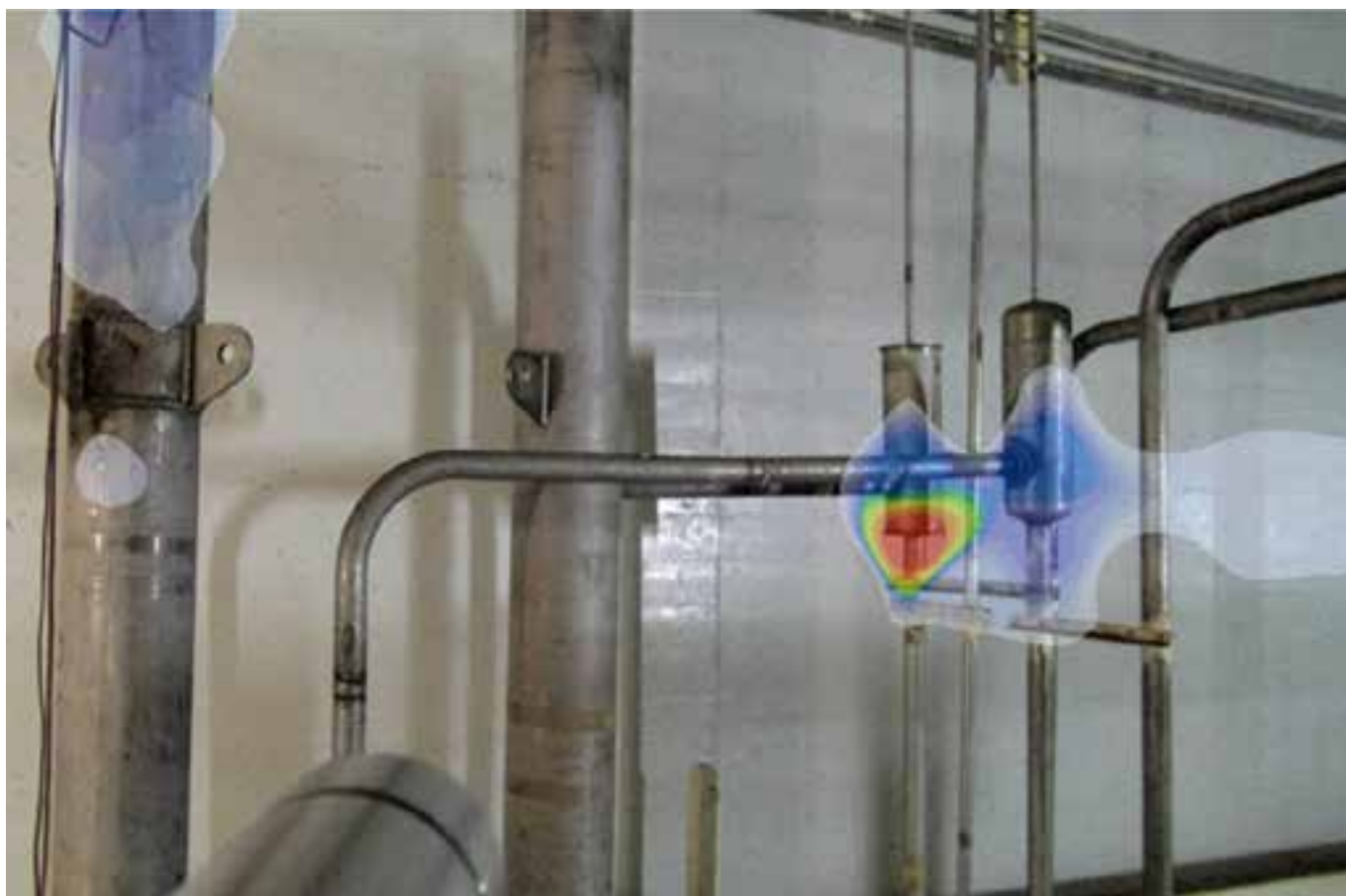
Hotspot located using a gamma imaging device
