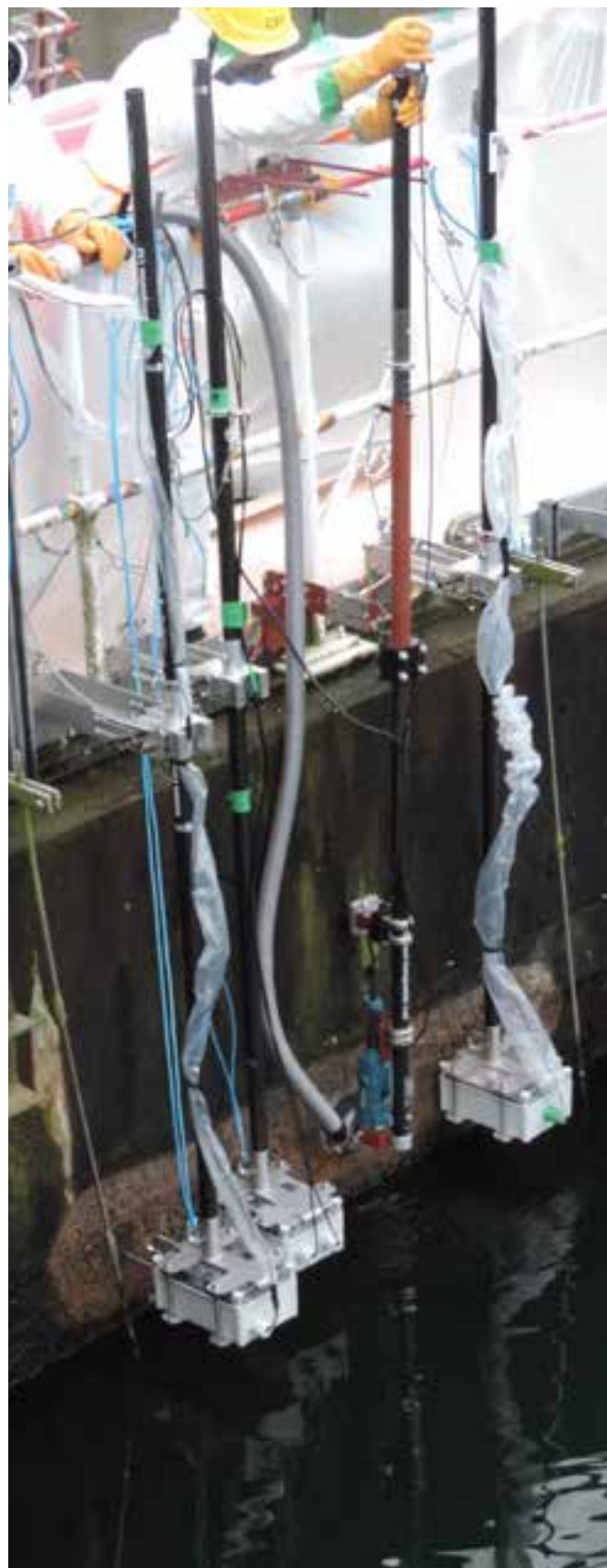
Deployment of radiometric equipment at a washed area of previously submerged concrete wall. Concrete planer also pictured.
