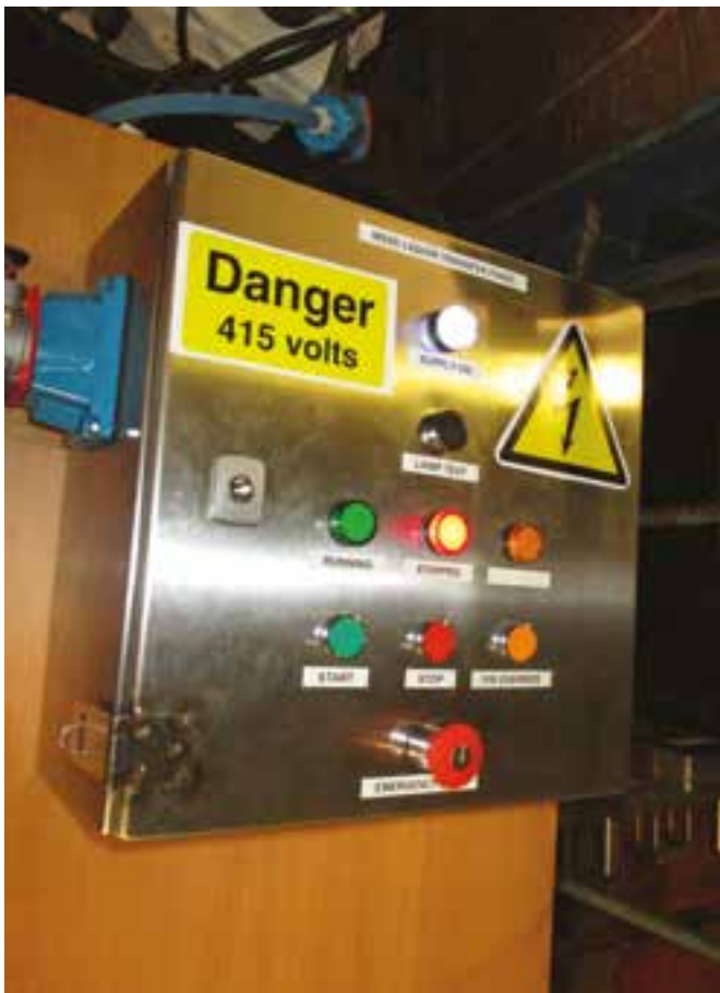
Pump control panel
