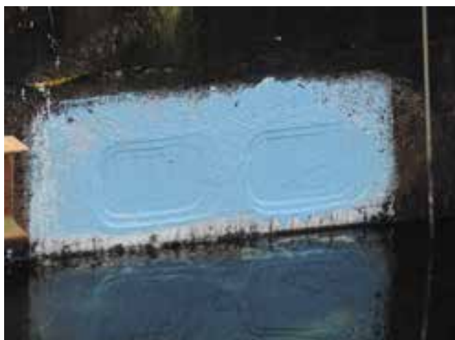
Epoxy sealant applied to PFSP pond wall (wall shaved at 3mm, 6mm and 9mm). White undercoat followed by a blue top coat.
