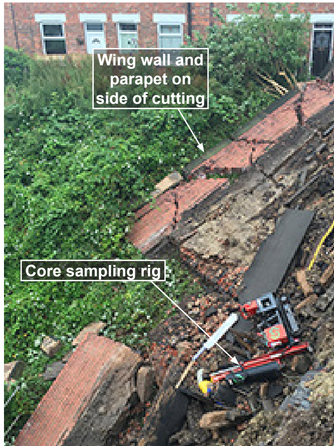
Figure 3: Masonry rubble post-incident (image courtesy of Network Rail)
