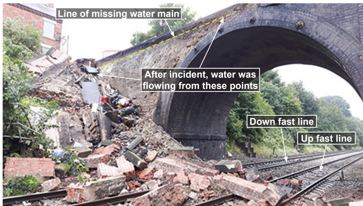
Figure 4: Extent of collapse and rubble obstructing the up and down fast lines
