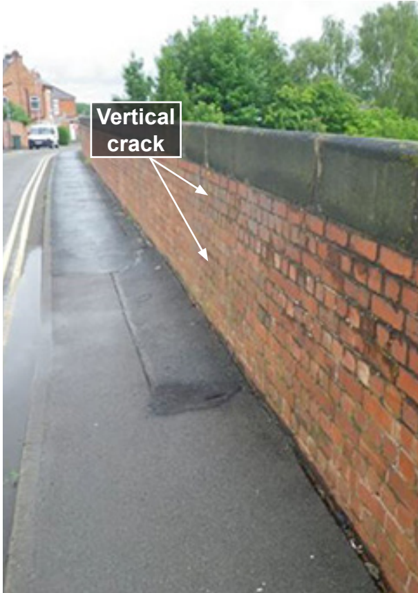
Figure 6c: June 2014 - the level of the footpath has been reinstated following the excavation in January 2012, but has continued to sink at the kerbside (image courtesy of Network Rail)
