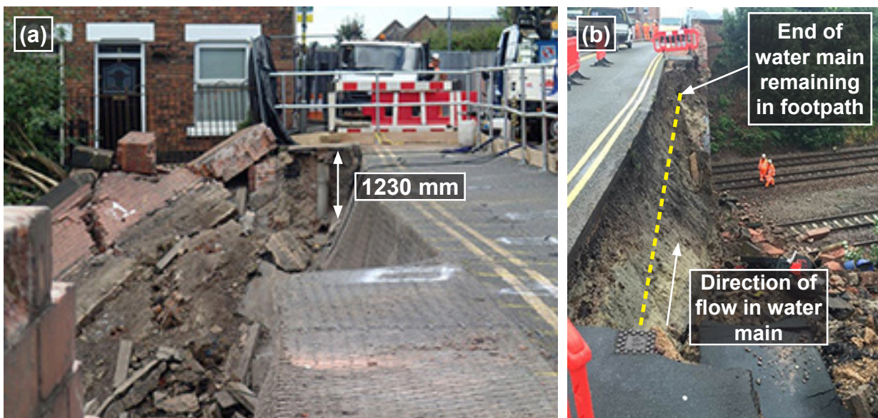
Figure 9: (a) exposed sluice valve and depth of water main; and (b) alignment of water main in footpath (image courtesy of Network Rail)
