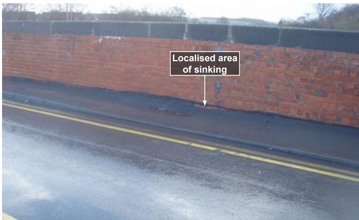
Figure 6b: January 2012 - subsidence continuing, with dips evident at both the parapet and the kerb (image courtesy of Network Rail)
