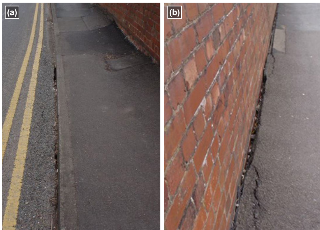
Figure 12: (a) March 2016 - void at kerbside; (b) May 2012 - gap opened up between footpath and parapet (images courtesy of Network Rail)
