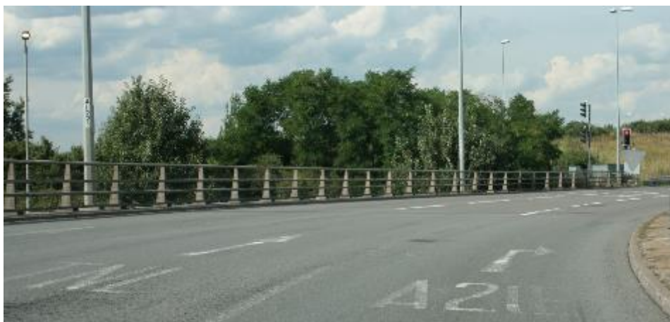
Figure 3-7 Faded Markings at A2/A282 Junction
