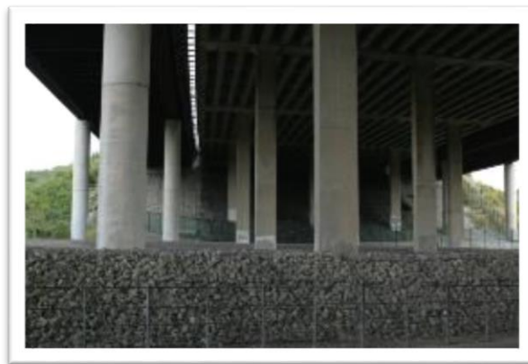
Figure 5-3 New hard landscaping under the Littledale viaduct, with the new A2 eastbound entry slip road clearly visible to the upper left of the picture.
