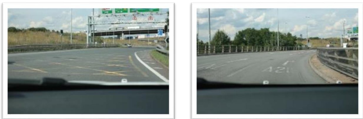
Figure 5-8 Typical examples of the faded road markings at the M25 Junction 2 roundabout; yellow box markings (left), and directional/ lane markings (right).
