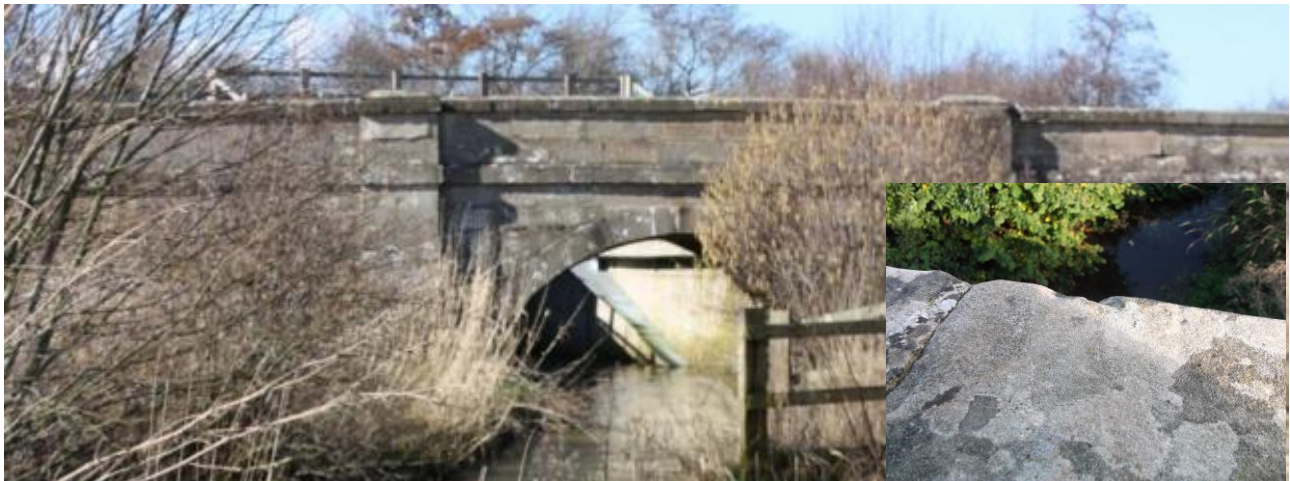
Figure 5.27 – Healam Bridge including inset photograph of wear due to historical line fishing on the bridge parapet (main photograph taken in March 2014)
