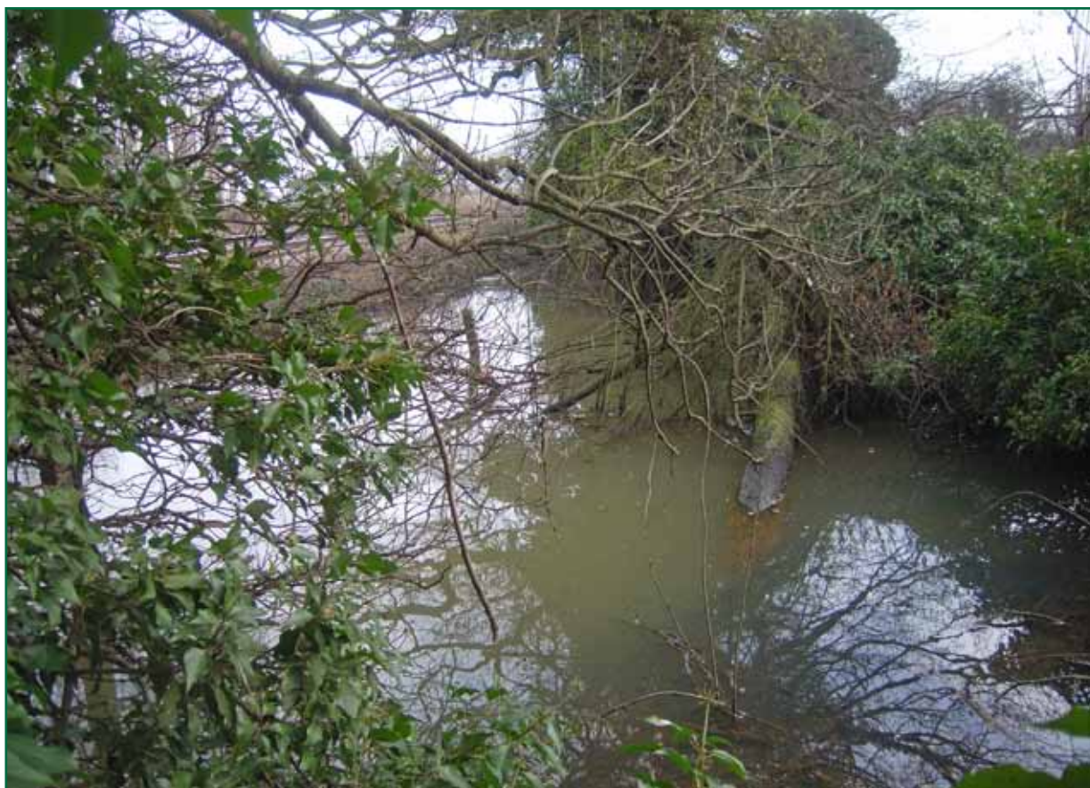
Figure 7: Water pooled next to the down line's cess
