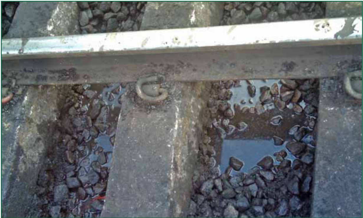
Figure 8: Water under the cess rail (photograph courtesy of Network Rail)
