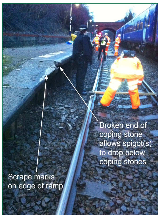
Figure 10: Witness marks on southern ramp
