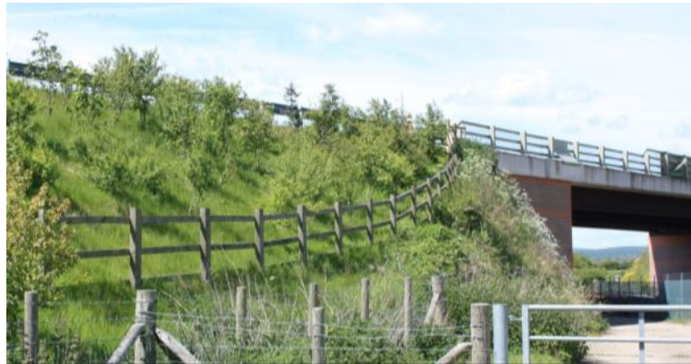
Figure 5.6 – Mitigation Planting at the Railway Bridge (poor growth)
