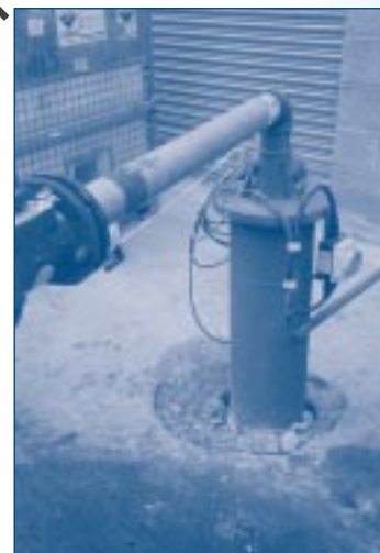
Above ground headworks (good practice) (still to be concreted at ground level), but sited close to stored chemical (bad practice)
