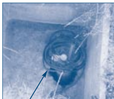
No grout behind casing
