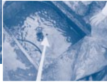
...resulting in contaminated drainage (oils and chemicals) flooding the chamber and polluting the borehole
