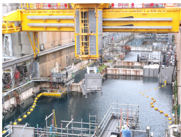
Progress on site decommissioning with the first bulk quantities of sludge removed.
