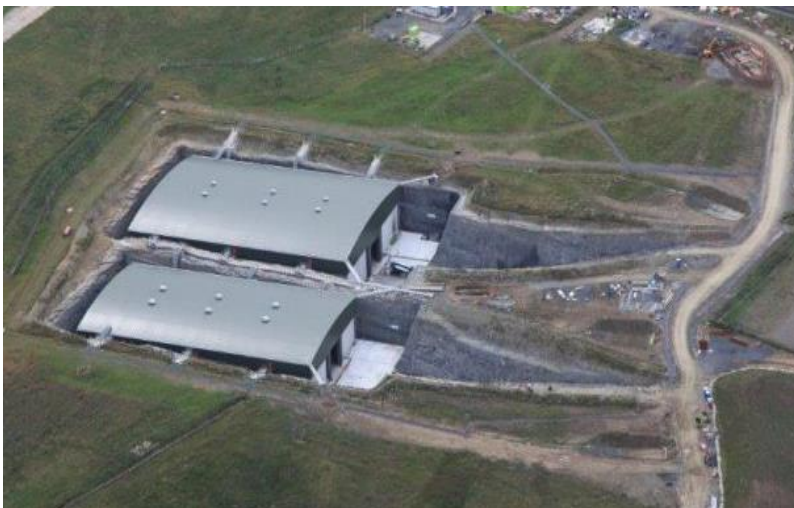
The first two vaults of the LLW Disposal Facility are now complete
