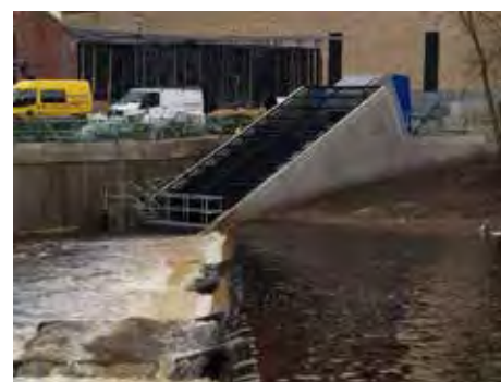
Hydro-power Archimedean screw turbine
