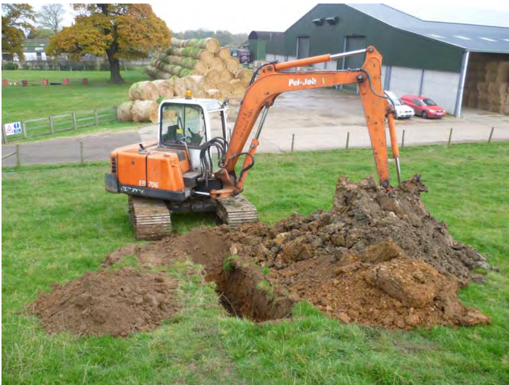
Plate 4 TP2 arisings – topsoil left, subsoil front right and Made Ground rear right.
