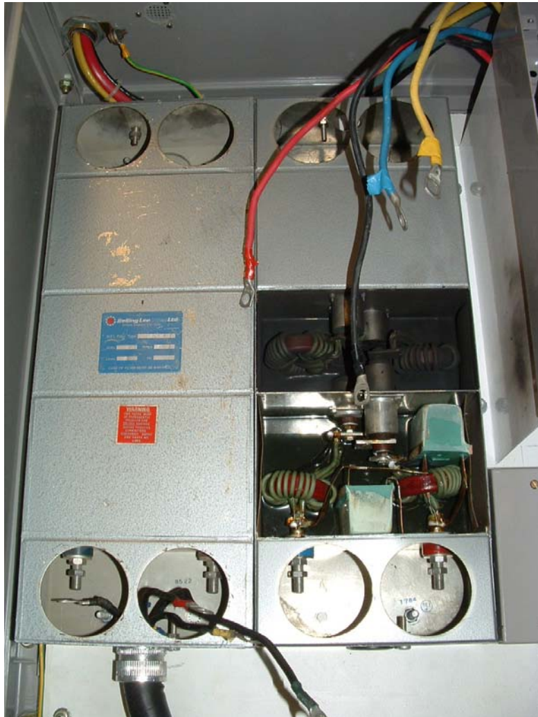
Figure 1: Damaged mains RF Filter in GRP Enclosure (note: cables have been disconnected).
