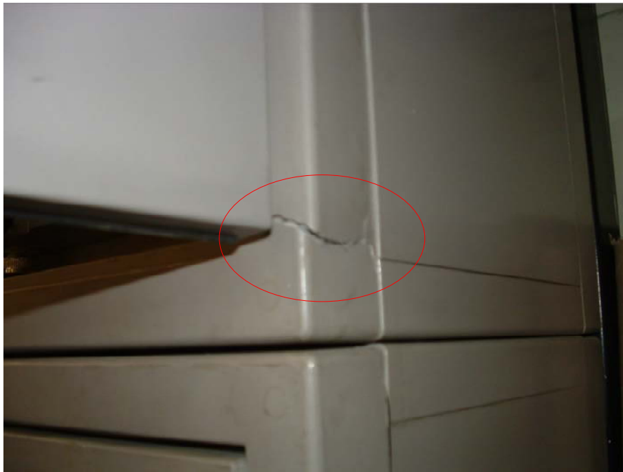
Figure 2: Damage to GRP enclosure.
