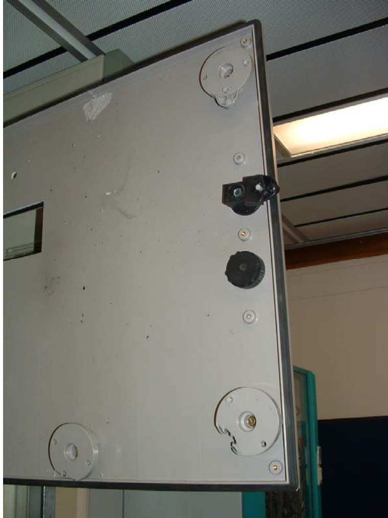
Figure 4: GRP enclosure door following the incident, note the interconnecting/latching bars were detached in the incident
