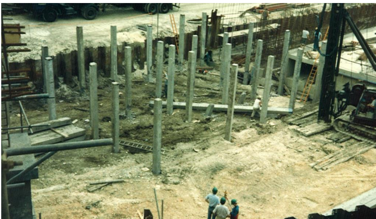
Construction Photograph 4. Upstream view, service tunnel within main building, piling for building.
