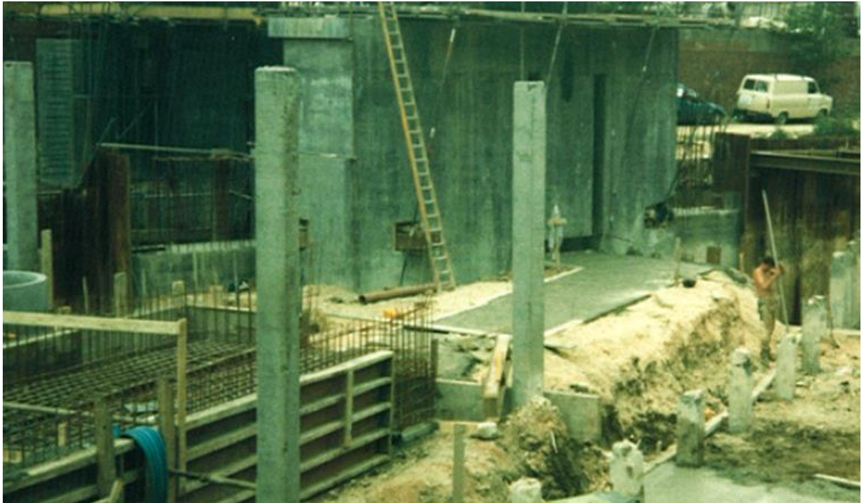
Construction Photograph 6. Downstream view, service tunnel formation between main building and barrier structure.
