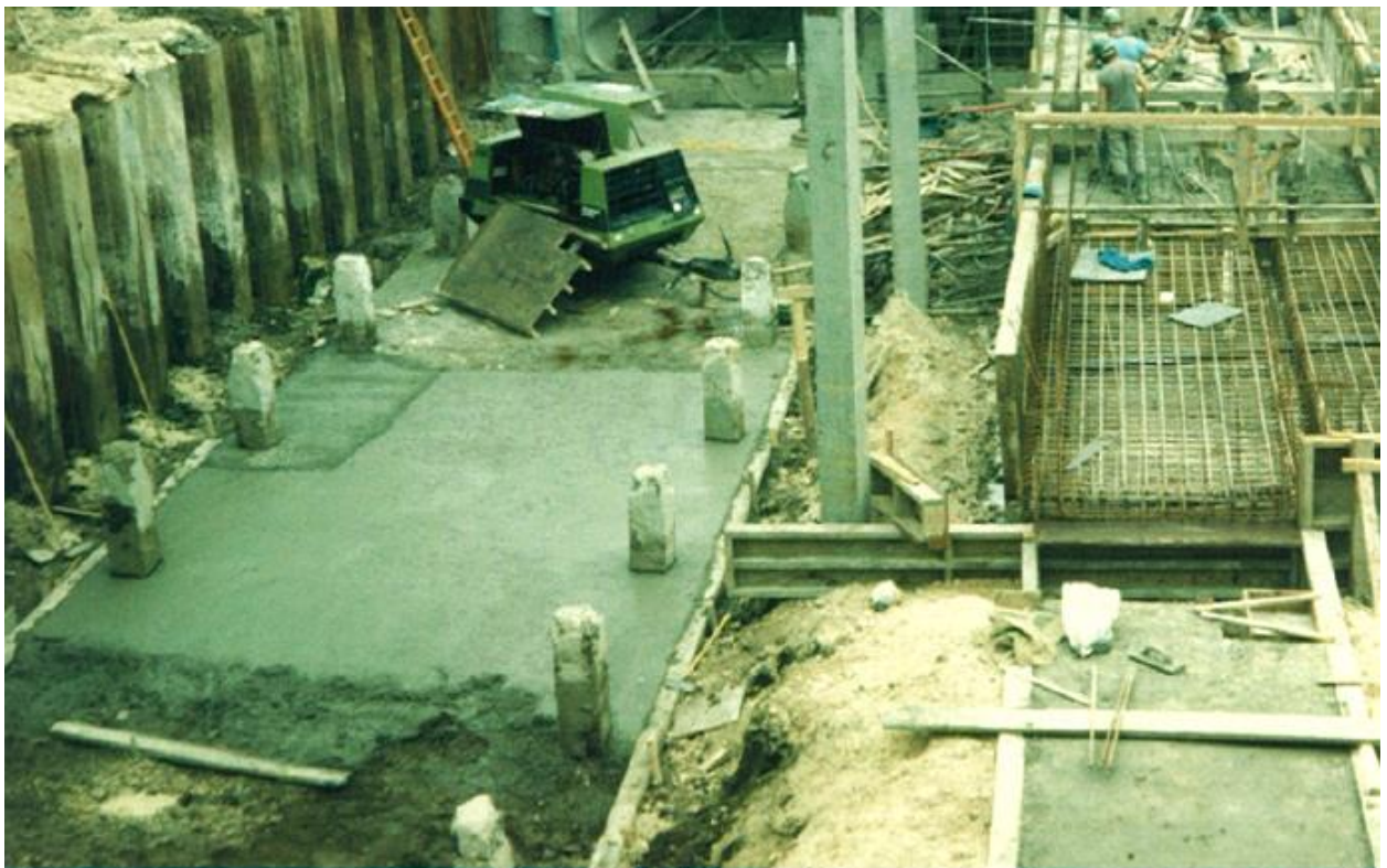
Construction Photograph 8. Upstream view, discharge culver blinding (left) and service tunnel right).
