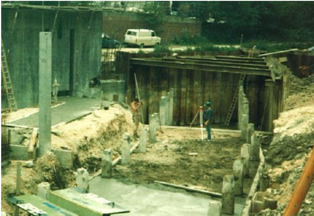
Construction Photograph 9. Downstream view, discharge culvert formation (right) and service tunnel (left).
