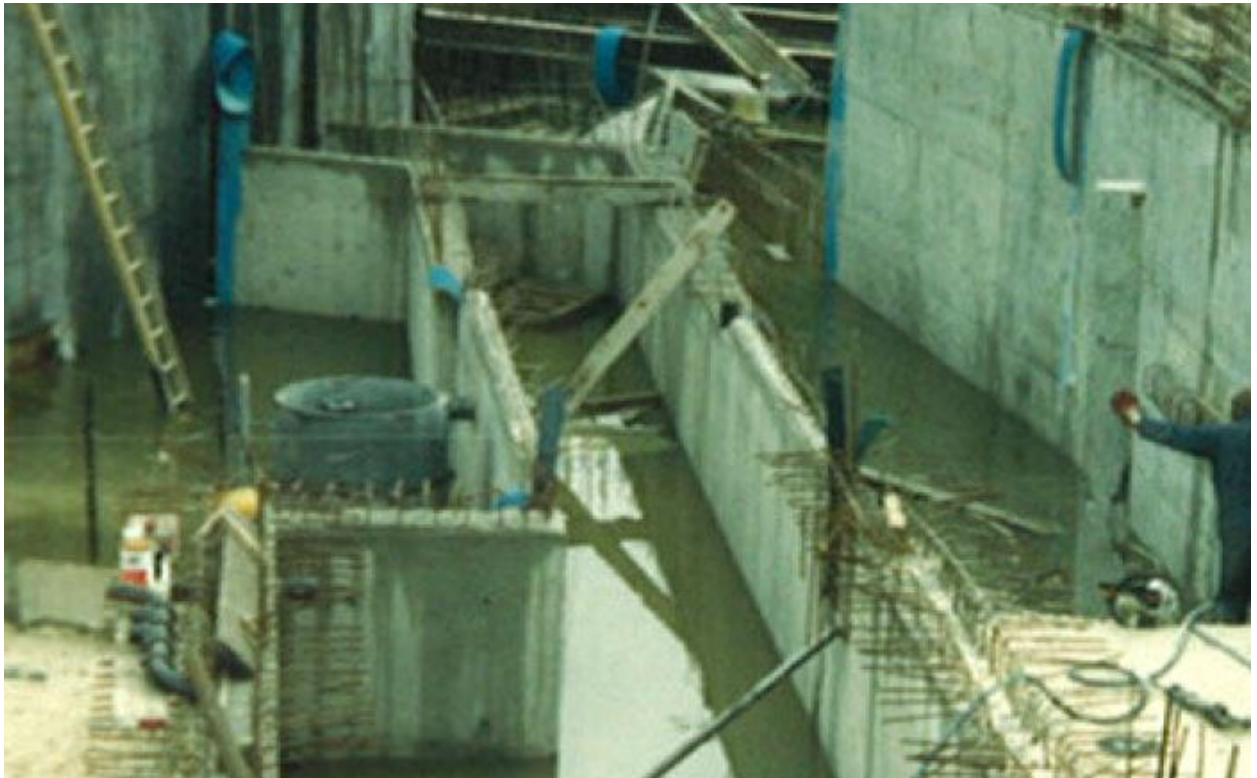
Construction Photograph 7. Downstream view, service tunnel between main building and barrier structure.
