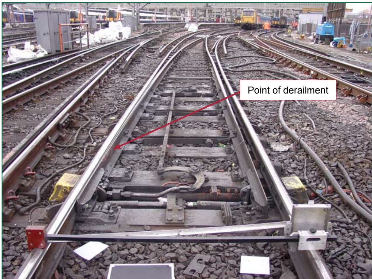
Figure 11: 1507 points viewed towards Waterloo station in the direction of travel. Train 1D54 is visible in the right background, with carriages 7 and 8 behind a Class 37 locomotive being used for recovery
