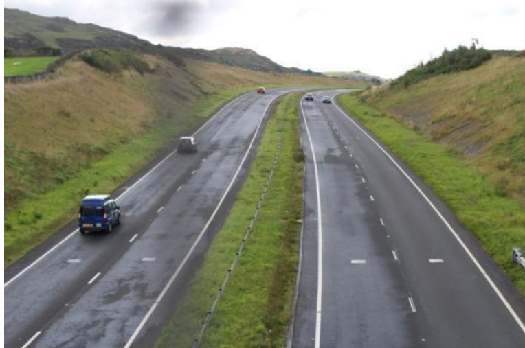
Figure 5.11 - View east from Oak Head over-bridge illustrating bare areas on cutting slopes September 2013
