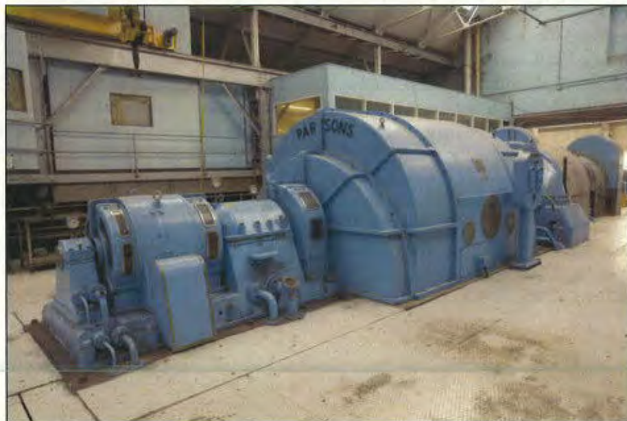
Fig 35. Renovating the 800 megawatt Al-Hartha powerplant 20km north of Basra was a much larger proposition.
