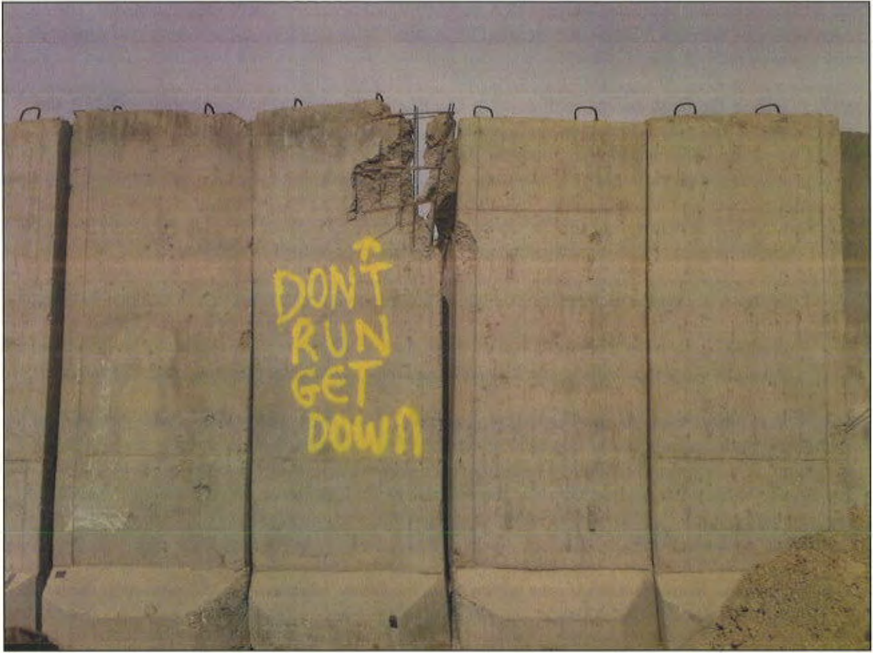
Fig 32. Wise advice. IDF damage to a jersey barrier.
