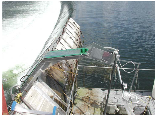
Figure 6.8. View of Chambly Dam eel pass from above. Note covers over the channel containing the substrate, and the electronic counting device on the pipe carrying the eels from the top of the pass to the keep net. Photo D. Desrochers.
