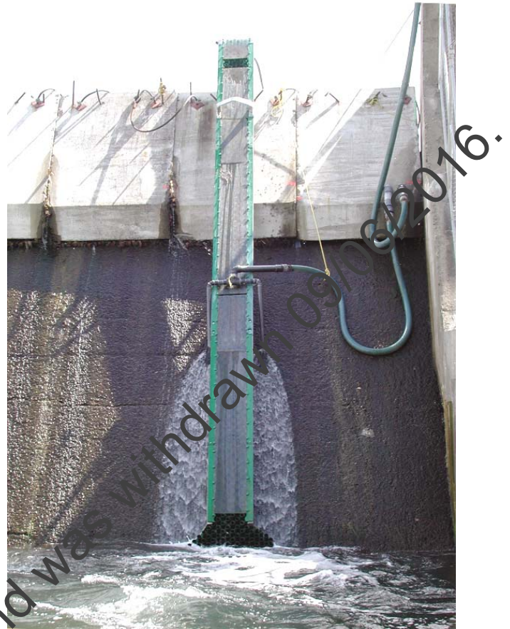
Figure 6.7. Eel pass at Chambly Dam. Note the breakwater blocks on the dam crest, and the gravity-fed attraction water being discharged from the two pipes part way down the dam face. Photo D. Desrochers.
