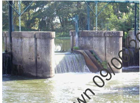
Figure 6.1. Eel pass at Moulin a Pigné
