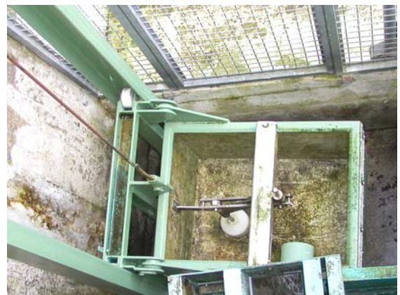
Figure 6.13. Lift hopper at Ville Hatte Dam eel lift in lower position.
