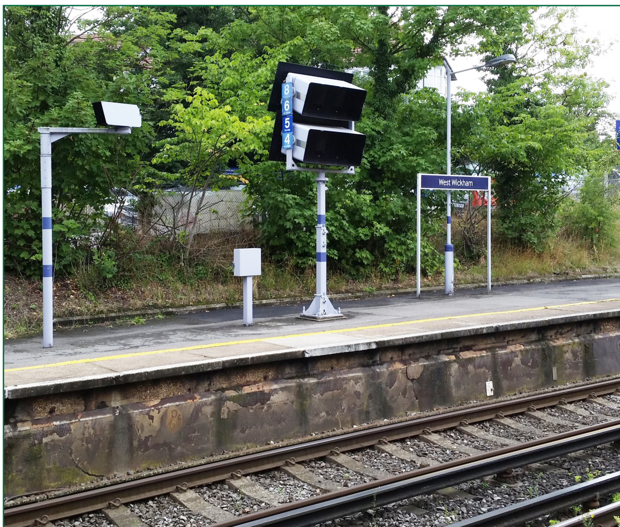
Figure 6: The eight vehicle monitor bank at West Wickham platform 2
