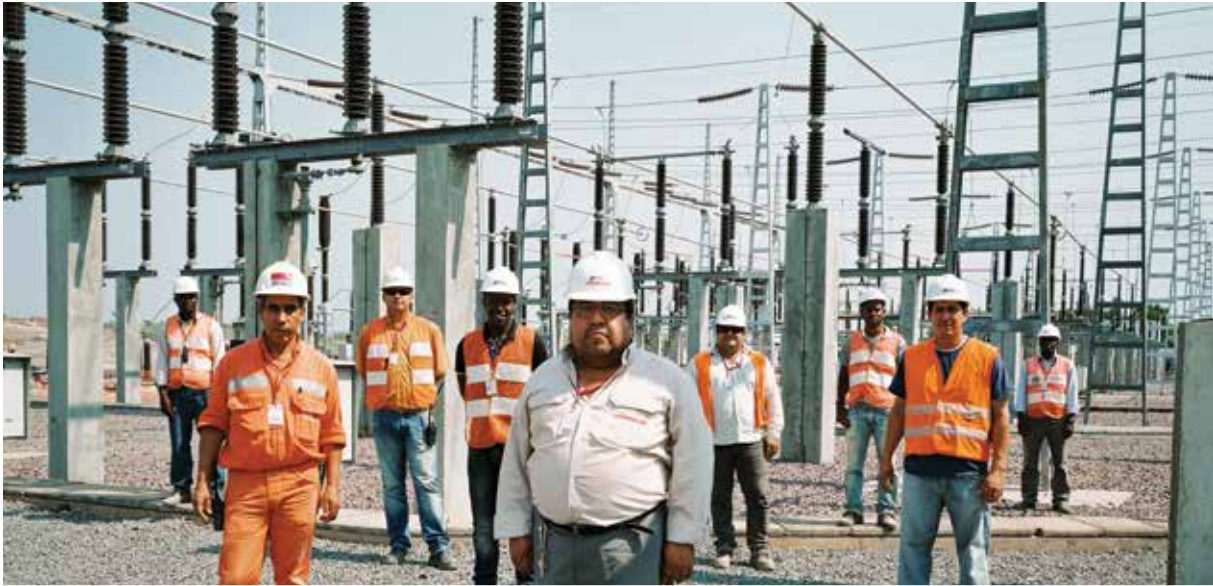
Employees of the Odebrecht Company, a Brazilian engineering firm, working on the renovation of the Cambambe dam and hydroelectric power station in Angola
