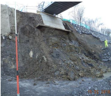
Steepened Cutting Slope Failure
