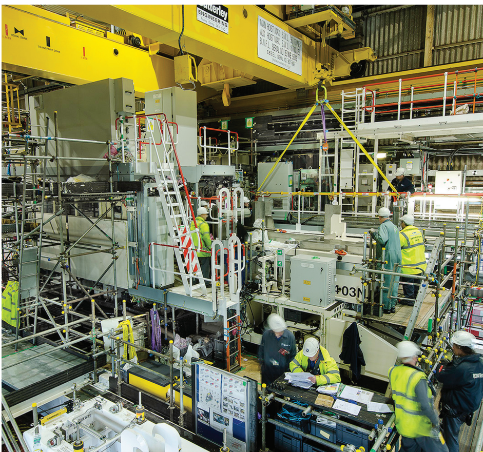
Photograph Below, the first Silo Emptying Plant is installed at the MSSS
