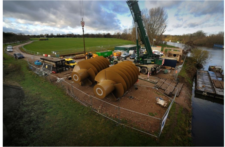
Two 40-tonne Hydropower turbines installed at the Environment Agency's Romney Weir on the River Thames.
