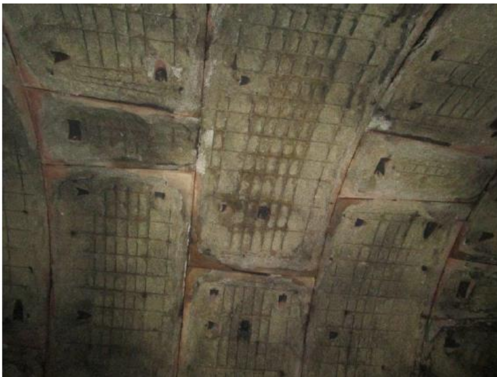
Figure 3: Damage to the tunnel above the burnt out lorries
