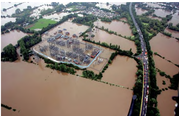
Walham during 2007 flooding
