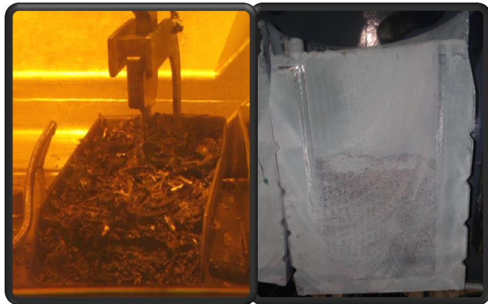
Increased throughput of the Magnox Encapsulation Plant speeds up fuel reprocessing at Sellafield
