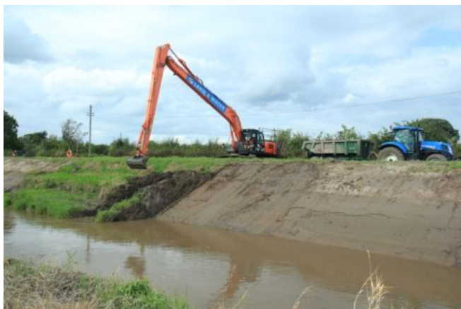
Work carried out on the Rivers Parrett and Tone following the winter 2013 to 2014 flooding
