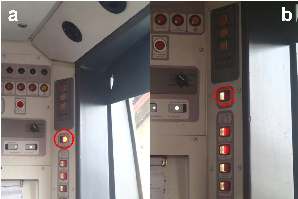
Figure 26: (a) Interlock light providing the driver with indication that the doors are closed and locked and (b) interlock not obtained
