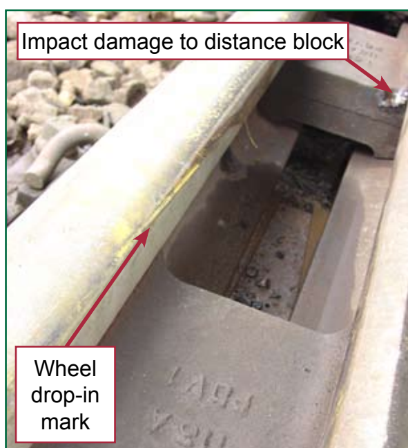
Figure 7: Point where wheelsets derailed
