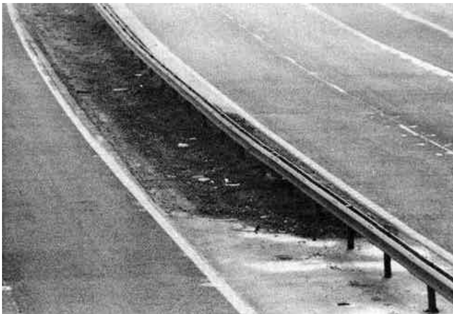
Photograph 2.13-1: Tensioned, Double Sided, Metal, Corrugated Safety Fence
