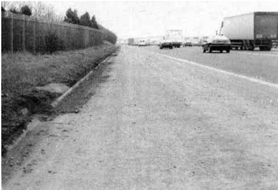
Photograph 3.12-2: MUCK - Excessive muck
