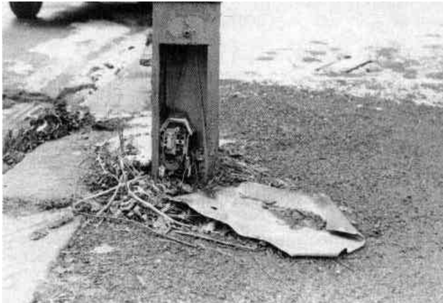
Photograph 3.19-2: EXPW - Exposed wiring
