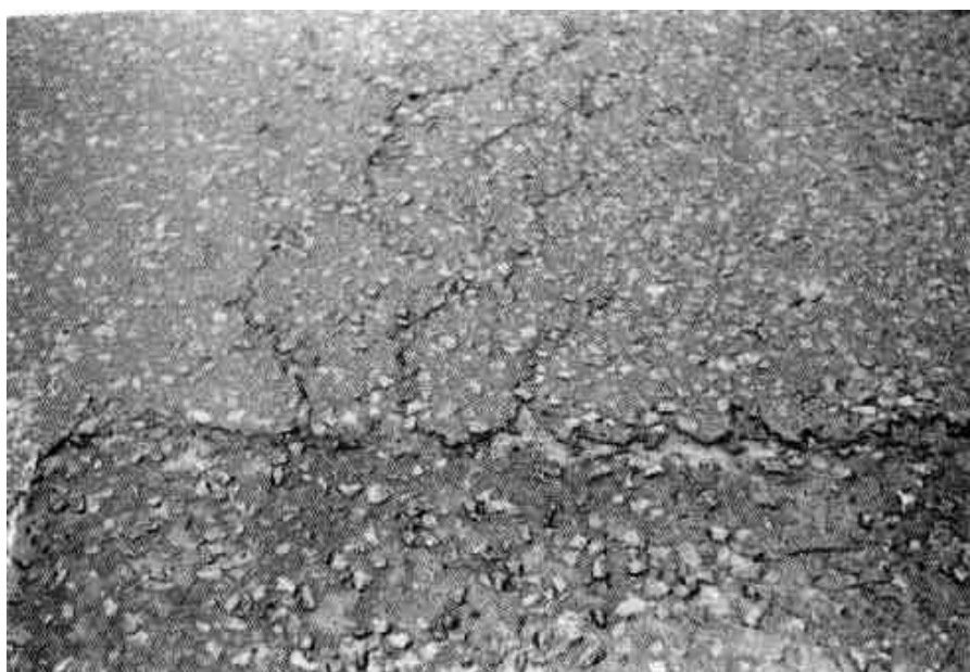
Photograph 3.3.1-8: TACK - Trench RI - adjacent cracking
