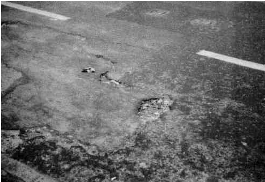
Photograph 3.3.1-6: PLMT - Patch - loss of material
