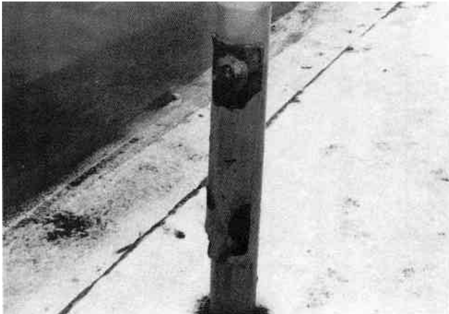
Photograph 3.19-4: DAMG - Damaged post / column
