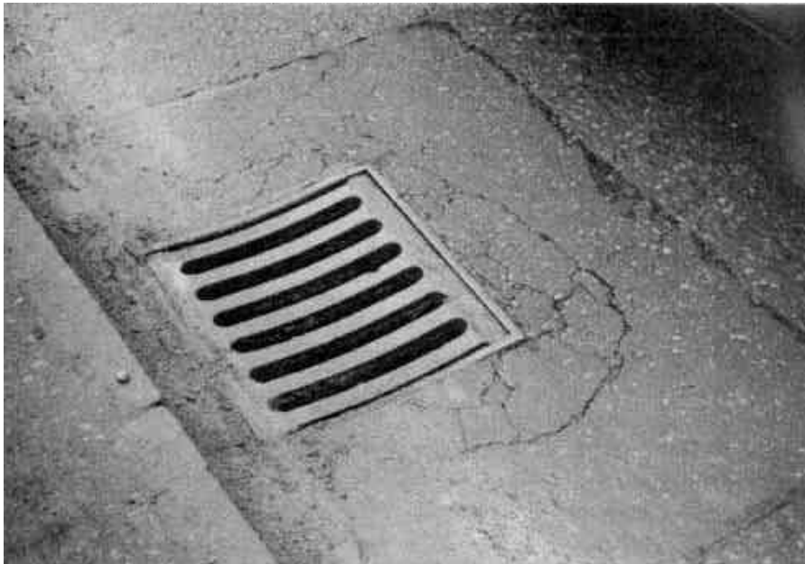
Photograph 3.3.1-4: CKIR - Cracking around ironwork
