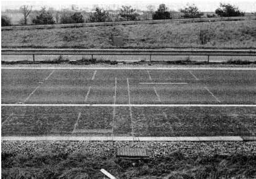
Photograph 2.8-3: Detector Loop (Traffic Counter)
