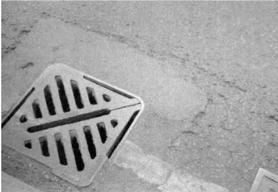
Photograph 3.3.1-5: PACK - Patch - adjacent cracking
