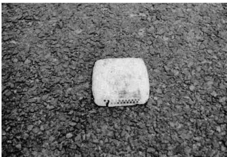
Photograph 3.15-4: DAMS - Damaged stud
