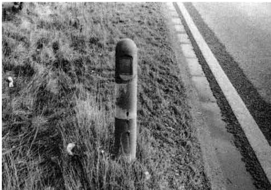
Photograph 3.17-5: COPT - Physical condition of post
