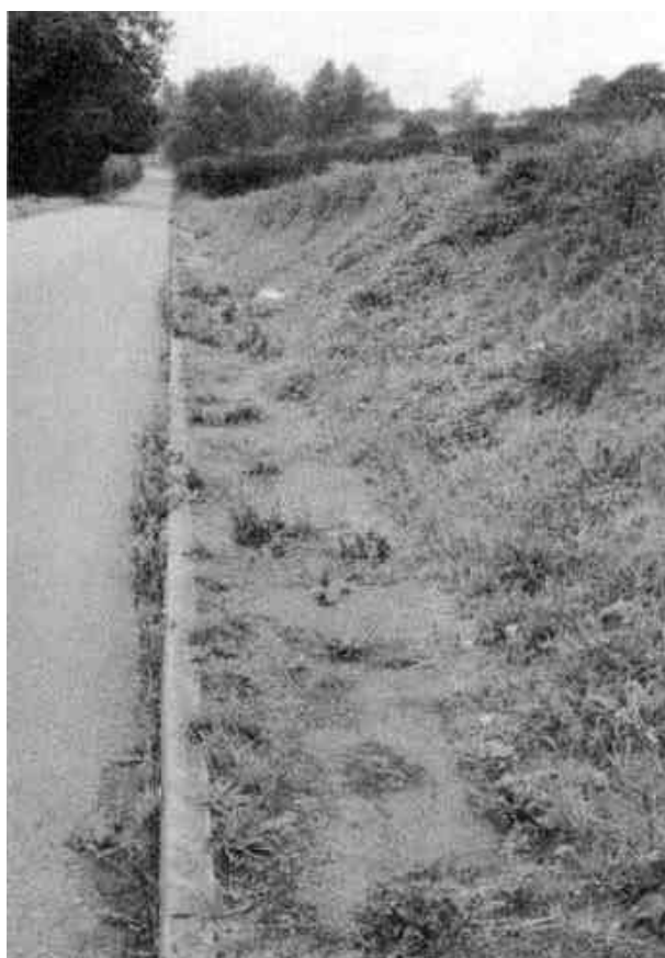
Photograph 3.4-10: OGVV - Overgrown by vegetation
