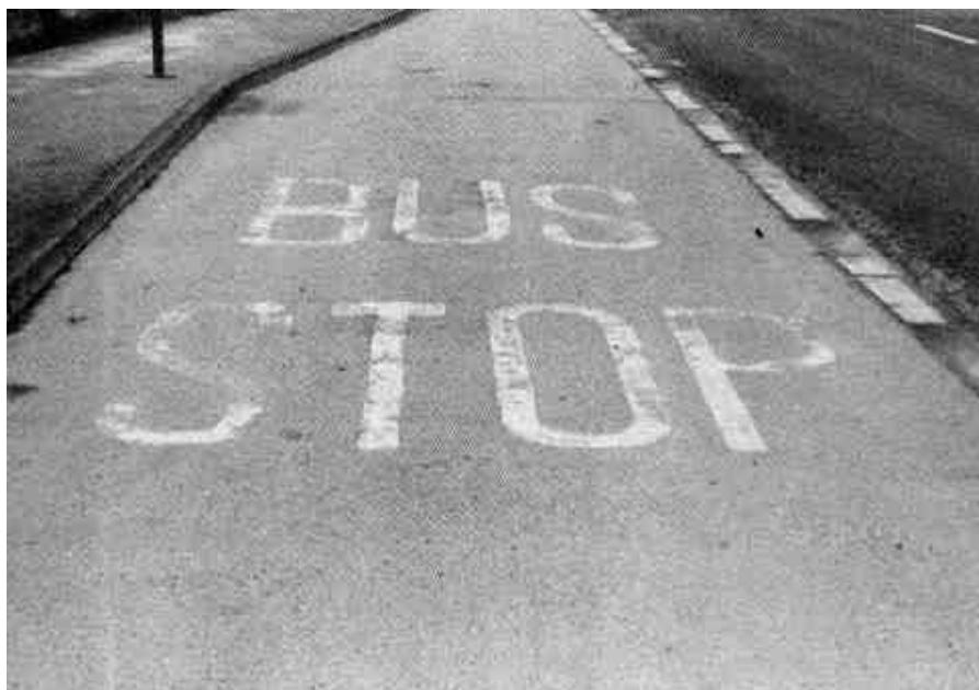
Photograph 2.16-11: Transverse and Special Road Markings - Words
