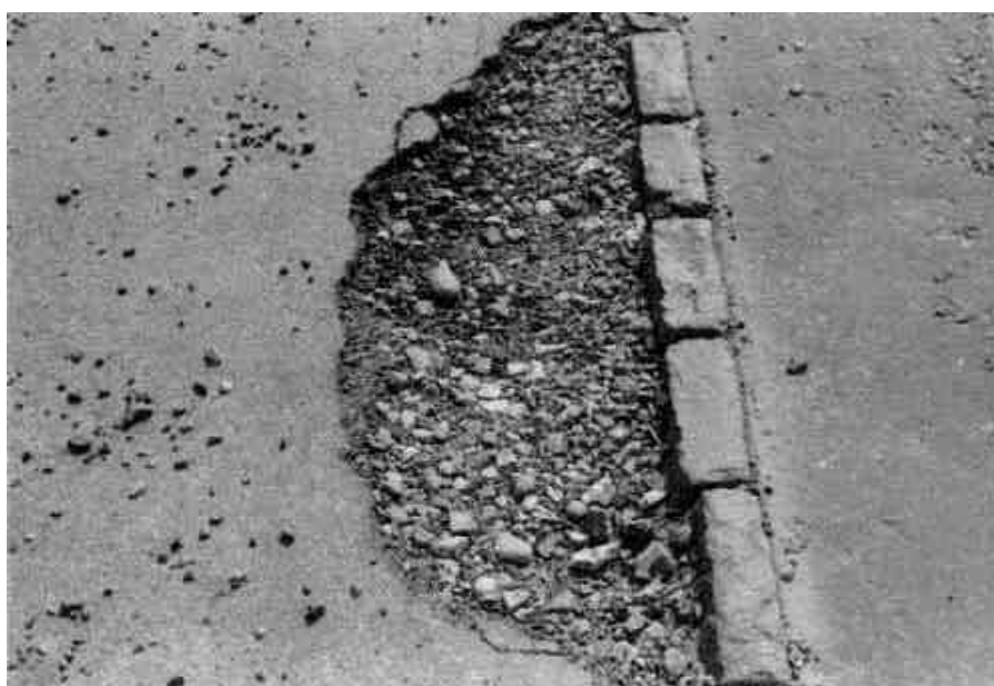
Photograph 3.4-4: BPOT - Black top - pothole
