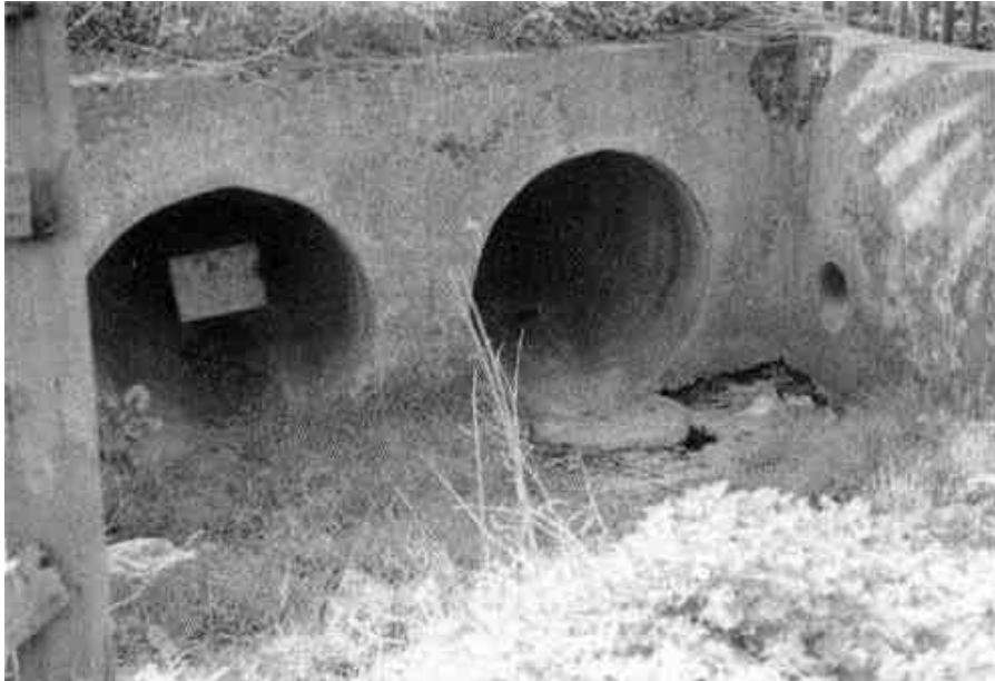
Photograph 3.7.7-1: FRFL - Free flow impeded
