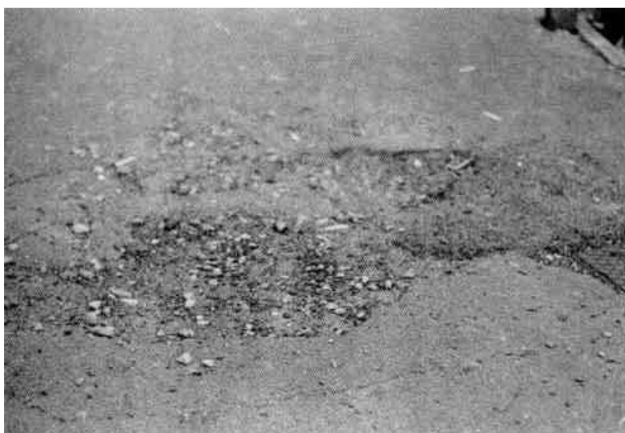
Photograph 3.4-8: FLMT - Failed patch - loss of material
