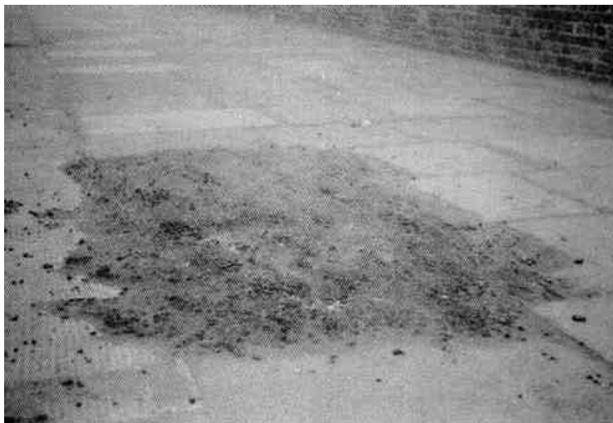
Photograph 3.4-9: FDLV - Failed patch - difference in level
