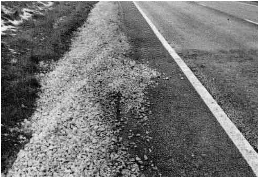
Photograph 3.7.6-2: FMDS - Filter material displaced
