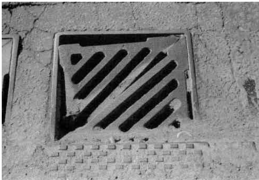
Photograph 3.5-3: IBCK - Cracked or broken
