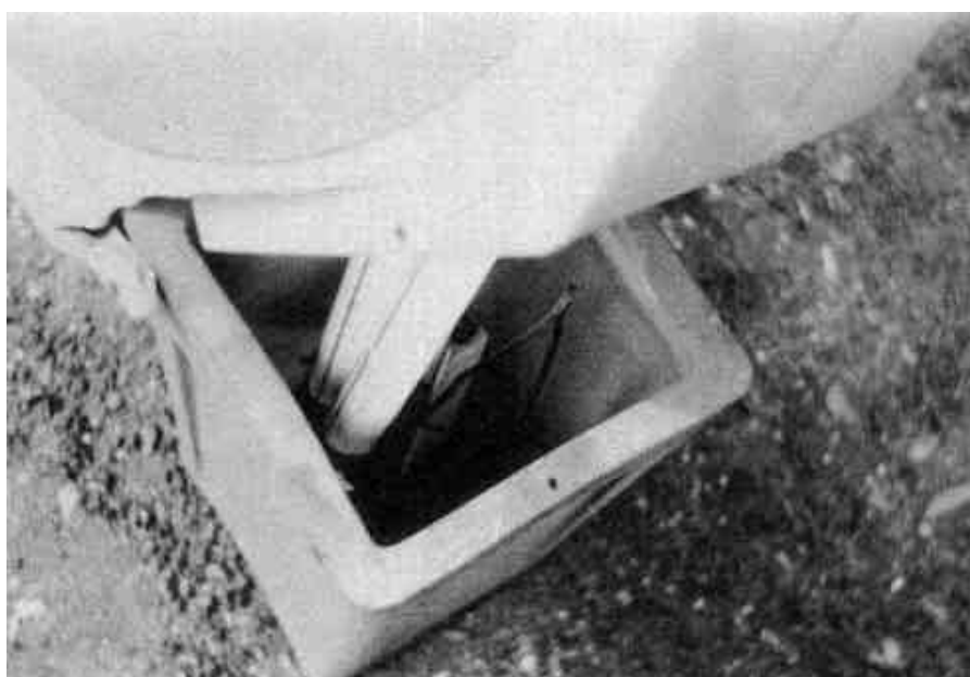
Photograph 3.17-6: EXPW - Exposed wiring
