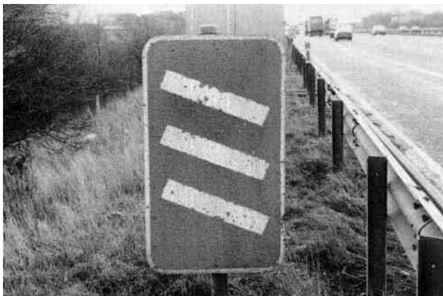
Photograph 3.17-1: SFLM - Initiate surface luminance check
