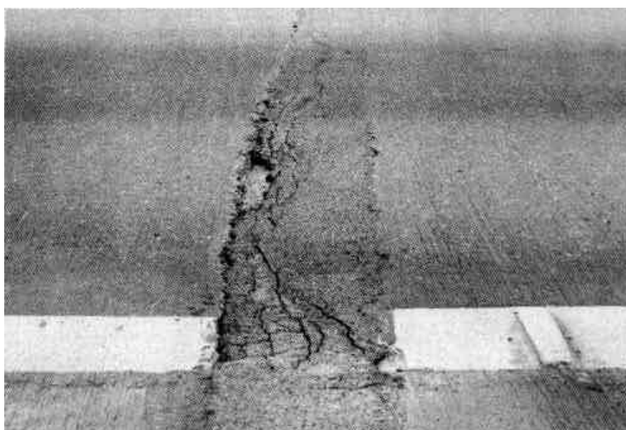
Photograph 3.3.2-8: RFAL - Failed repair
