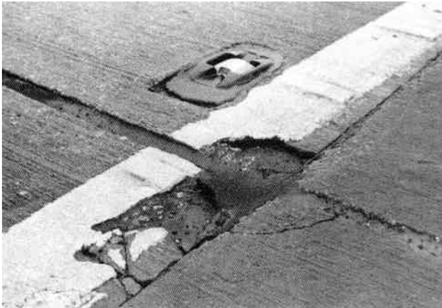
Photograph 3.3.2-3: DSPL - Deep spalling at joints
