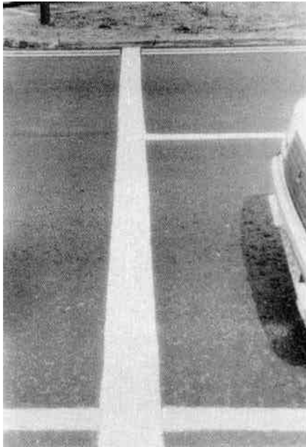
Photograph 2.16-9: Transverse and Special Road Markings - Stop
