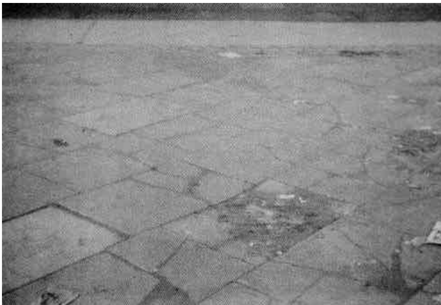
Photograph 3.4-2: SLCK - Slab cracking
