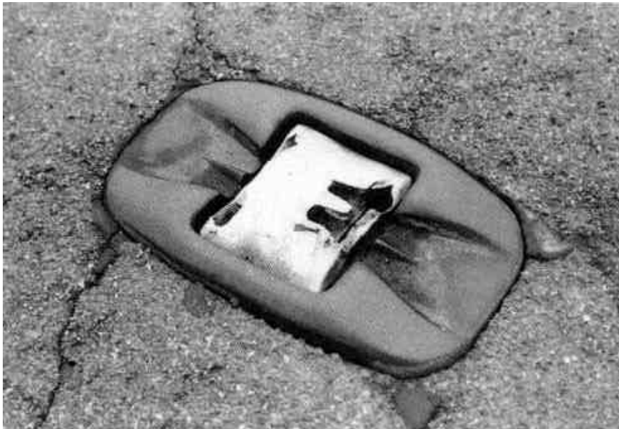
Photograph 3.15-6: MISR - Missing reflector
