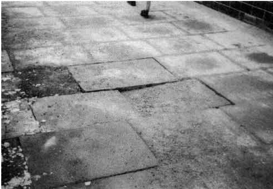
Photograph 3.4-1: SLPF - Slab Profile - uneven/trips/gap > 20mm
