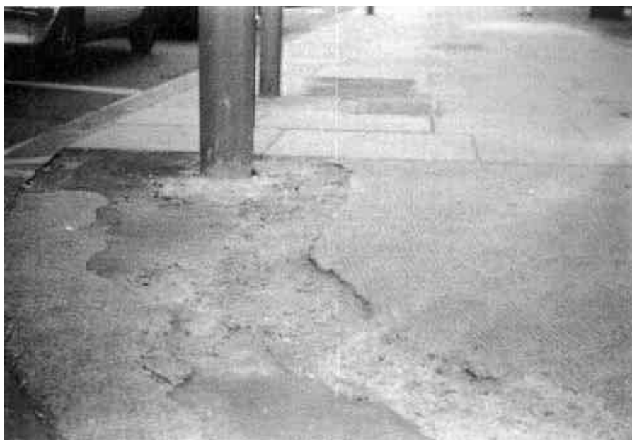
Photograph 3.4-11: RLMT - Trench RI - loss of material
