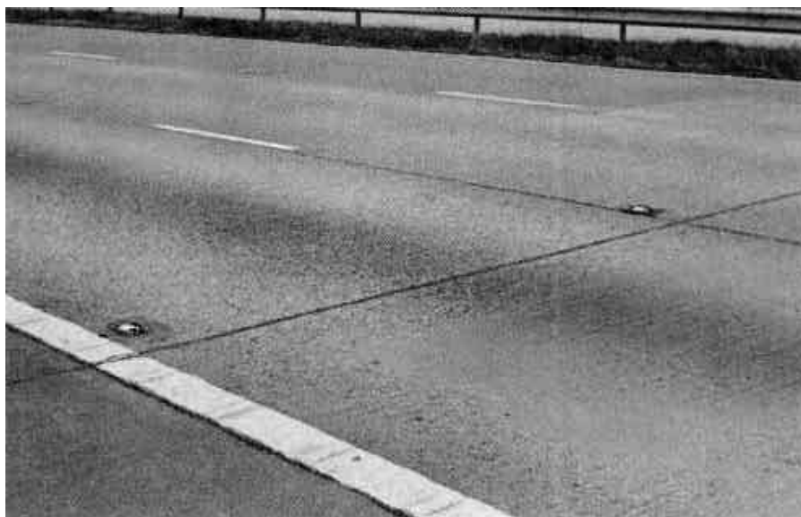
Photograph 3.3.2-7: SRTX - Surface texture worn
