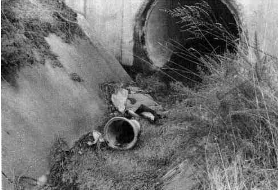
Photograph 3.7.5-3: DRUB - Deposited rubbish
