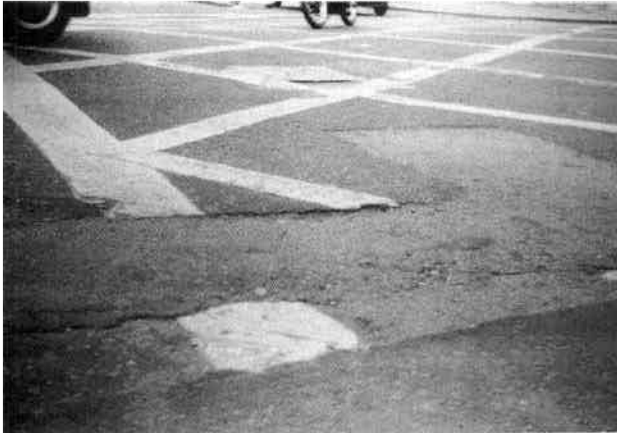
Photograph 3.3.1-9: TLMT - Trench RI - loss of material
