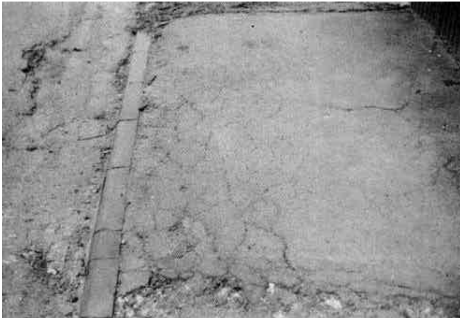
Photograph 3.4-6: BECK - Black top - extensive cracking
