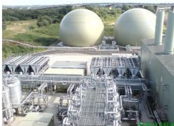
Figure 16 SBAP at Davyhulme WwTW
