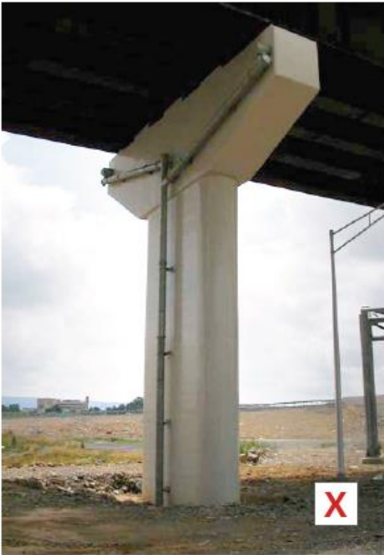
Viaduct rainwater collection: exposed rainwater collection pipes, ©Timothy Reichard / m-plex.com
