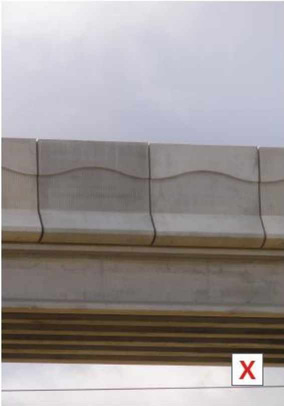
Pre-cast parapet panels: visible colour mis-match between adjacent panels, © Grimshaw
