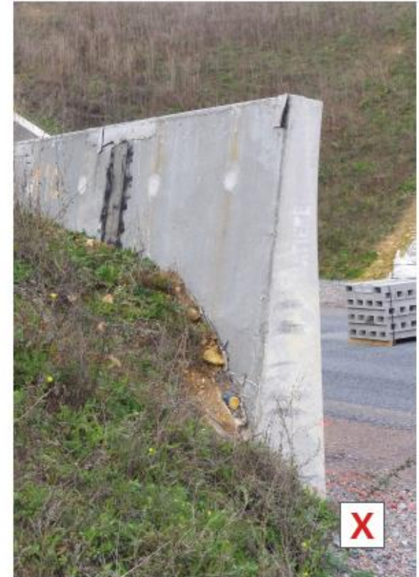
Pre-cast retaining wall panels: poor quality finish visible to rear, © Grimshaw
