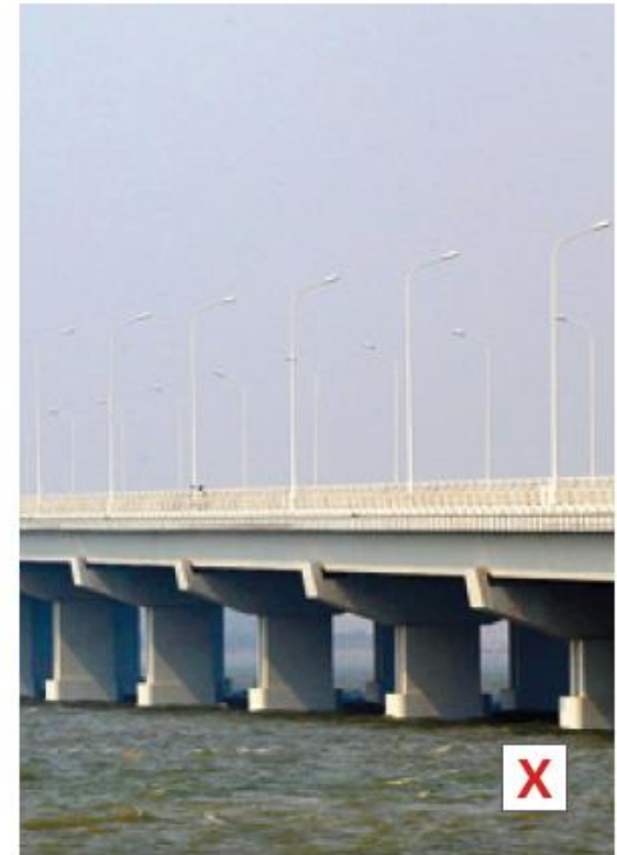
Exposed crossheads interrupt line of viaduct soffit, Pulandian Bay, China, © Jinzhou New District Information Center
