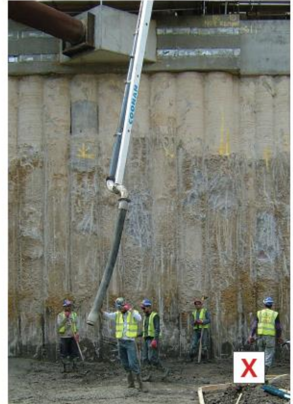
Secant pile embedded wall: not suitable for walls visible to the public, © Grimshaw
