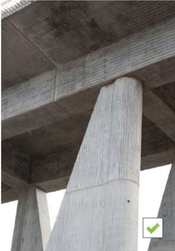
Concrete finishes: consistent finish used across all structural elements, © Schlaich Bergermann Partner
