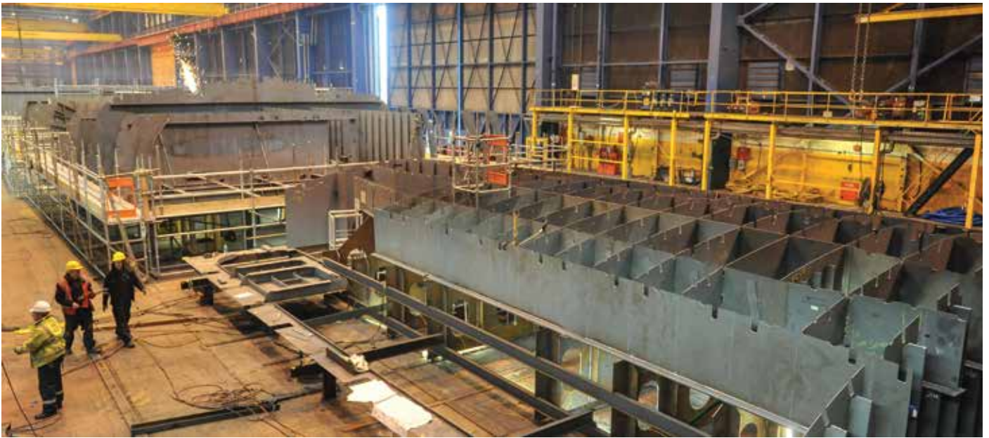
Under way: the first sections of the first OPV, HMS Forth , are pictured in Glasgow
